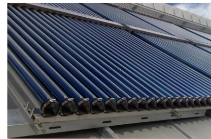
Example of Solar Thermal unit
