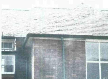
Figure 3: missing roof tiles in quad
