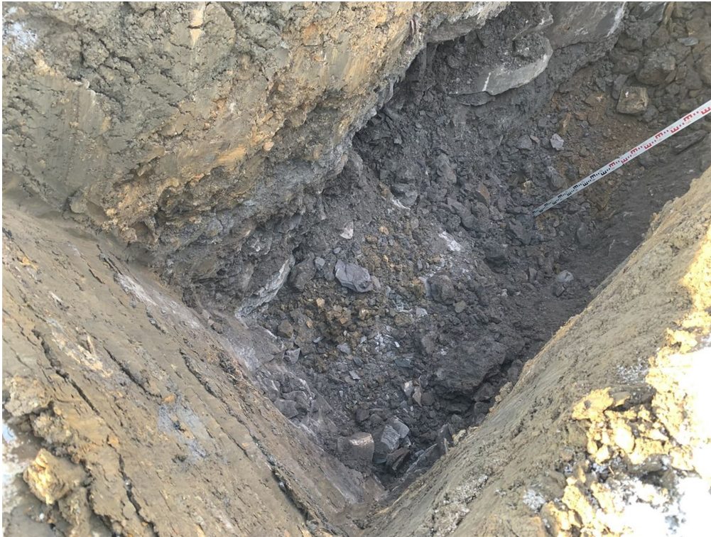
Photograph 11: Trial pit TP02. Southern face of trial pit, view from the south east to the north west.
