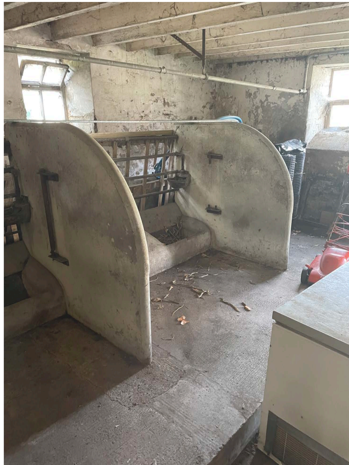
Photo Ref: E09 View of Nether Mill Barn (Internal Detailing Cattle Feeding Station)
