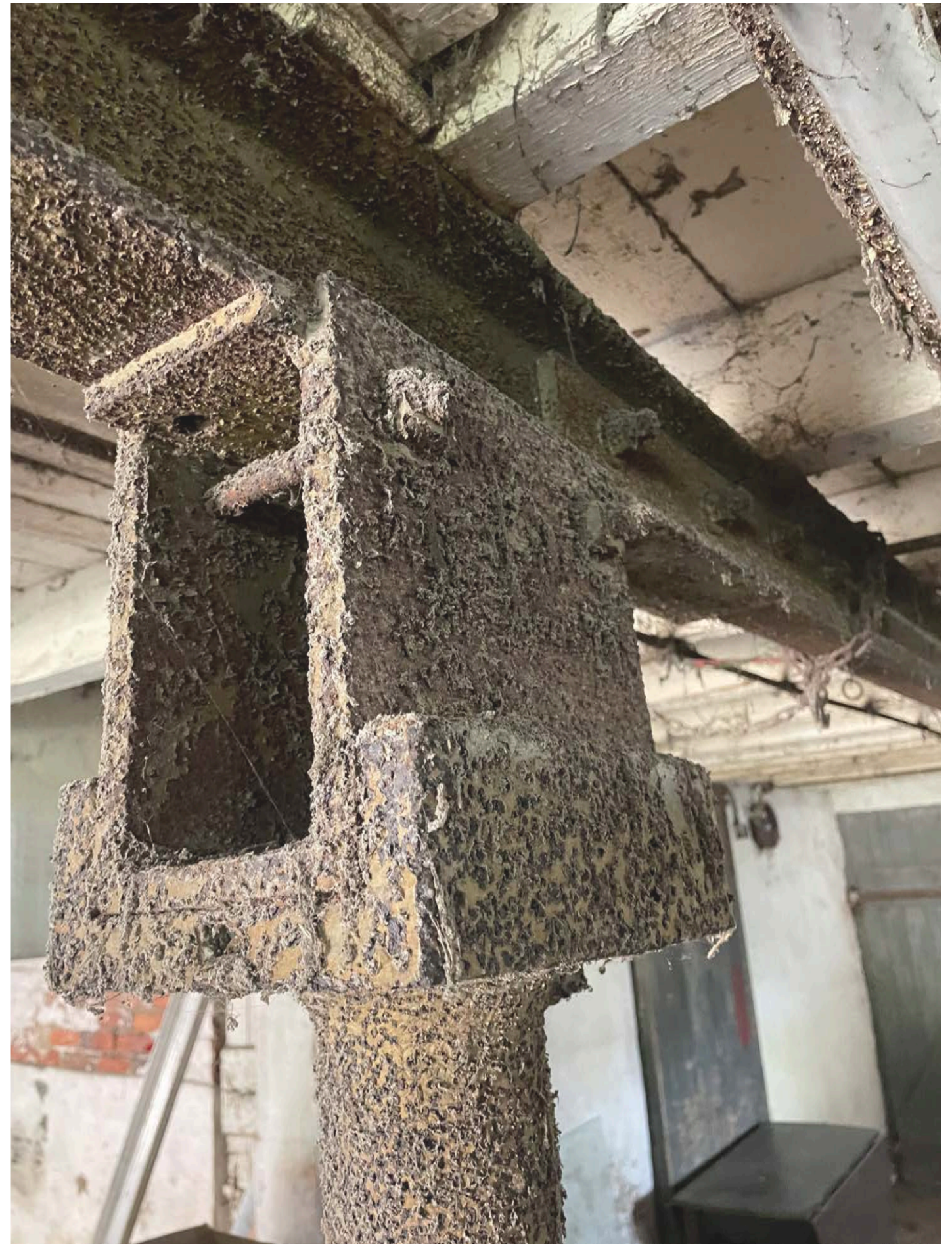
Photo Ref: E11 View of Nether Mill Barn (Internal Detailing First Floor Structure)
