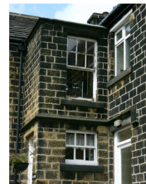
Traditional sashes with UPVC replacements to RHS
