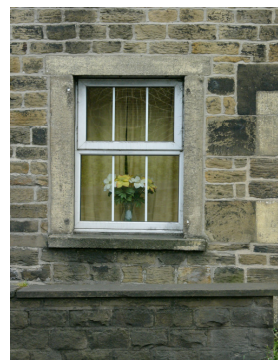
Unattractive modern glazing
