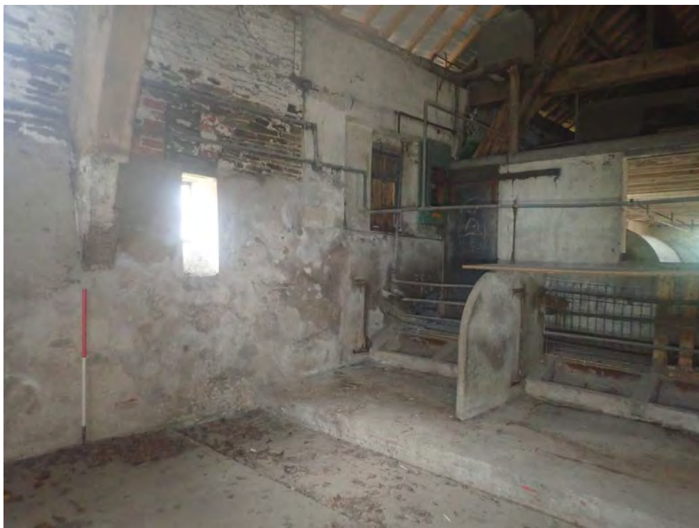
Photograph:40 Direction: N Digital Ref: NEMB2_0035 Description: Partially blocked cart door in Bay 2 NW wall.
