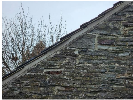
Photo 12 Example gaps along the verge
