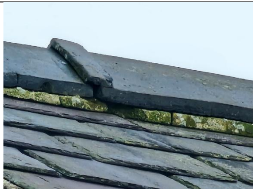
Photo 18 Gap under ridge tiles
