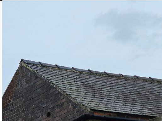
Photo 16 Shows gaps along the ridge
