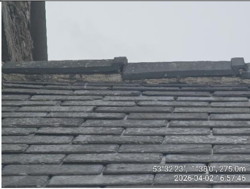
Photo 19 Gap under ridge tile
