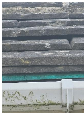
Photo 6 Example gap under concrete stone effect tiles
