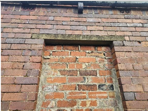
Photo 17 Gap under lintel
