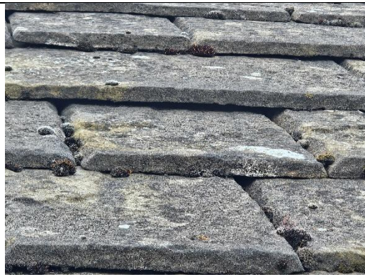
Photo 10 Example gaps under tiles
