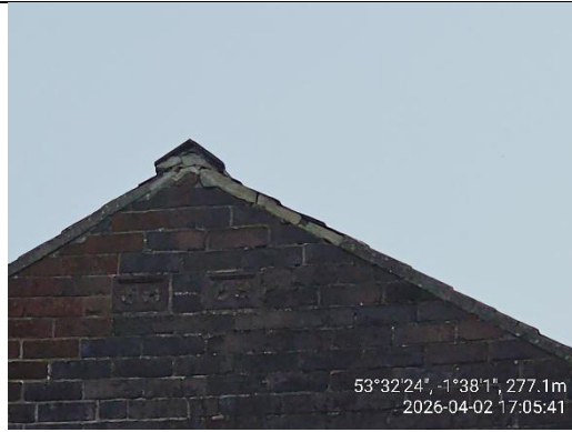
Photo 20 Gaps along verge
