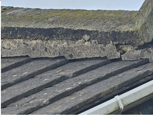
Photo 7 Example gap along base of gable parapets
