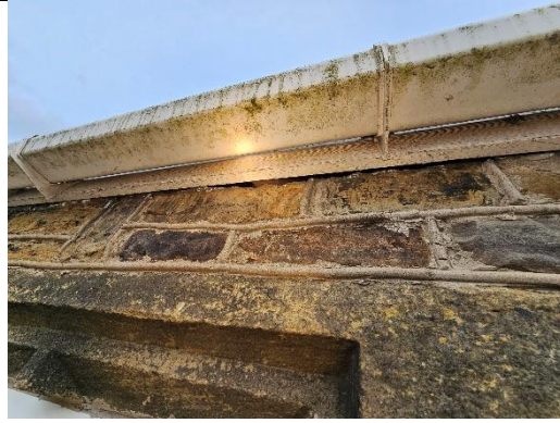
Photo 8 Gap under fascia
