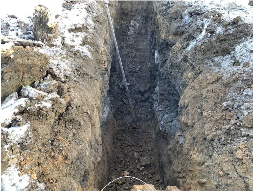
Photograph 03: Trial pit TP01. Eastern face of trial pit, view from the west to the east.
