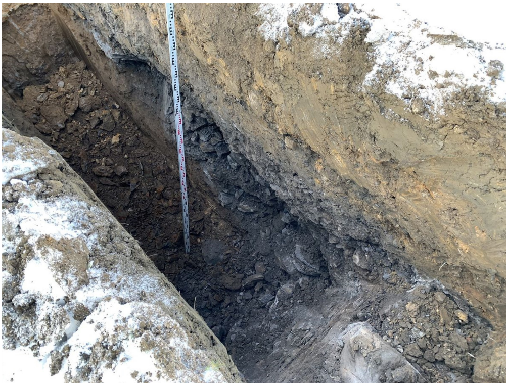
Photograph 04: Trial pit TP01. Northern side of trial pit, view from the south east to the north west.
