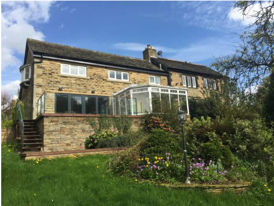
Fig 10 – Photo highlighting joint between new and old
