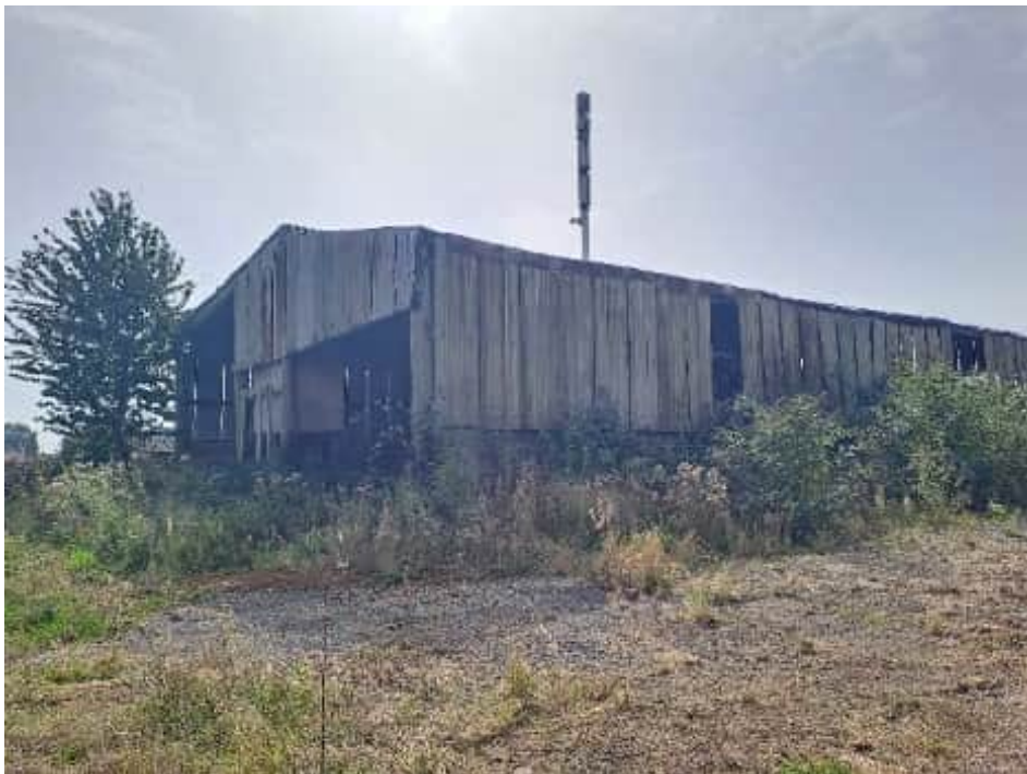
Plate A-2 – South view of another barn, timber frame, with breeze block base curtain walls, corrugated metal to upper walls and roof.
