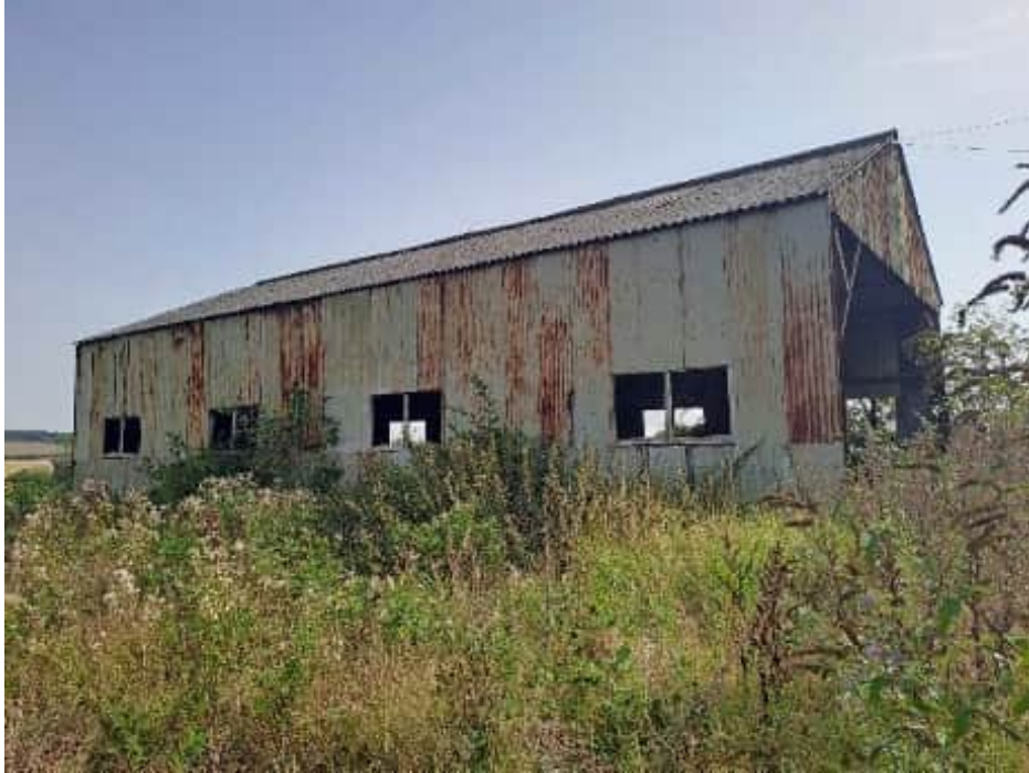
Plate A-1 – View looking east at the first metal barn. Combination of metal and wooded frame, clad with corrugated metal sheeting with an asbestos roof.
