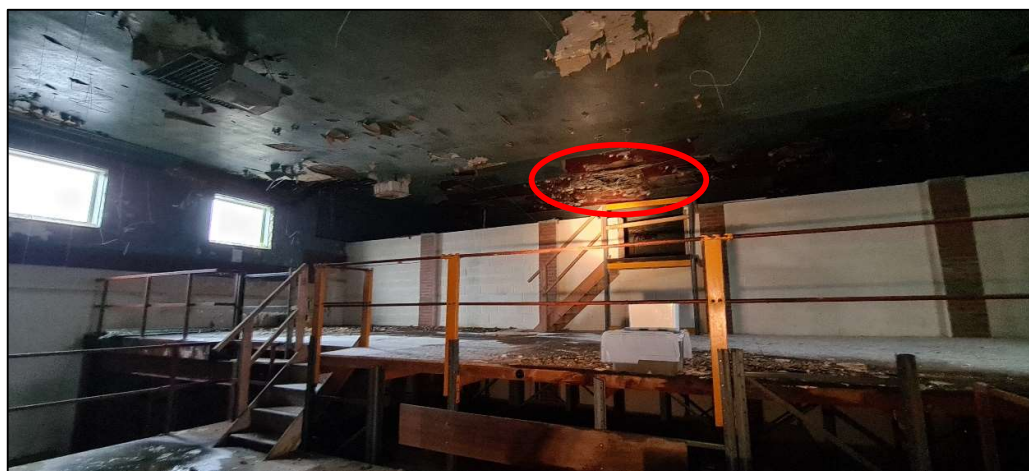
Plate 6. damaged ceiling with laths (circled red) visible
