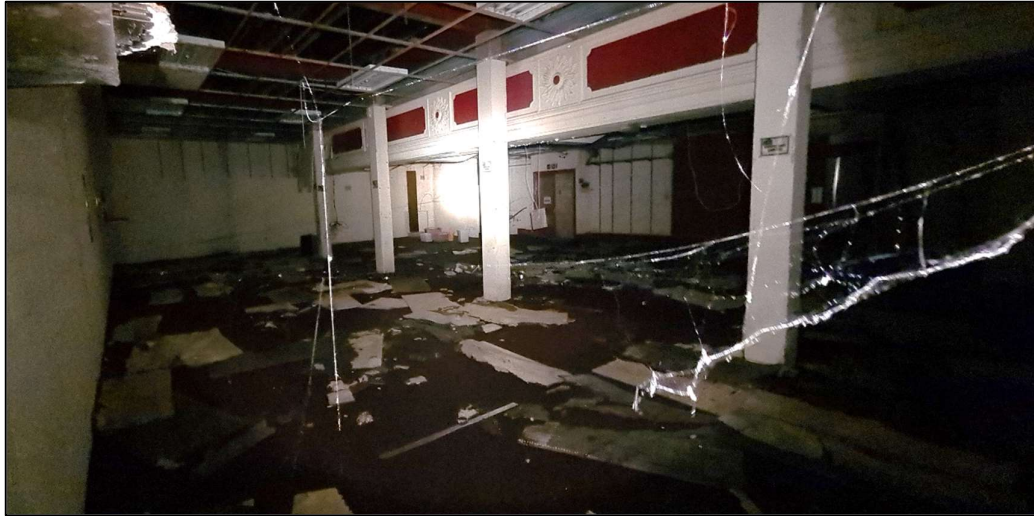
Plate 7. The foyer with very few suspended ceiling tiles remaining and hanging cobwebs shown
