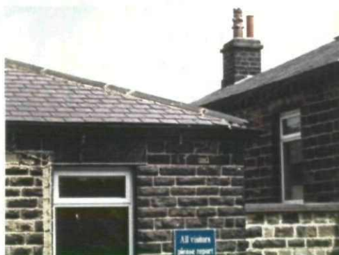
Figure 5: loose tiles, sixth form
