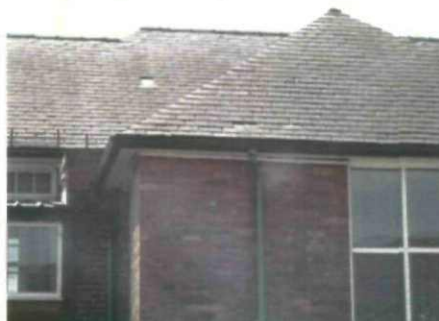
Figure 3: missing roof tiles in quad
