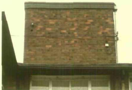
Figure 4: Gap in brickwork in water tower
