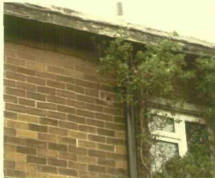
Figure 3: Gap in wall of caretakers house
