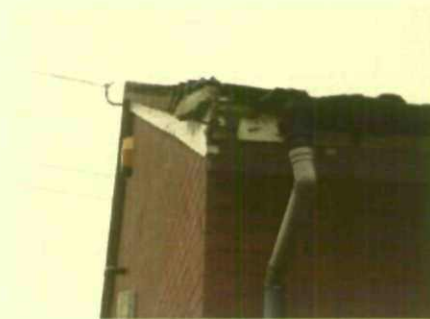
Figure 3: C - Block (kitchens), gap and missing/loose tiles
