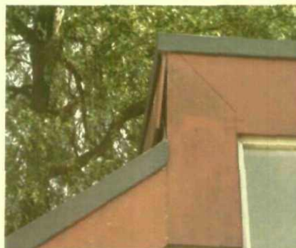
Figure 5: Loose Bargeboards, Technology
