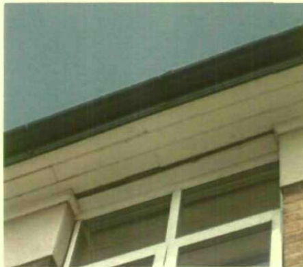
Figure 4: loose soffits at rear of main building
