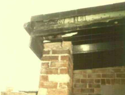
Figure 5: Loose soffits/bargeboards in the region of the I-T suite
