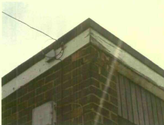
Figure 1: loose brickwork at corner of dining room
