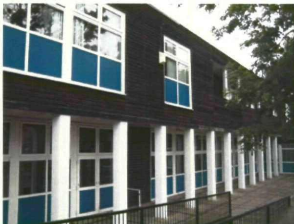
Figure 5: hole in fascia boards of main hall, eastern face
