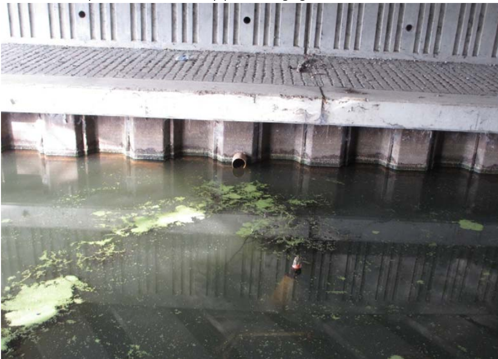
End of Highway drain into canal below A6195 approximately 200m south of site. Assumed To drain part of carriageway.
