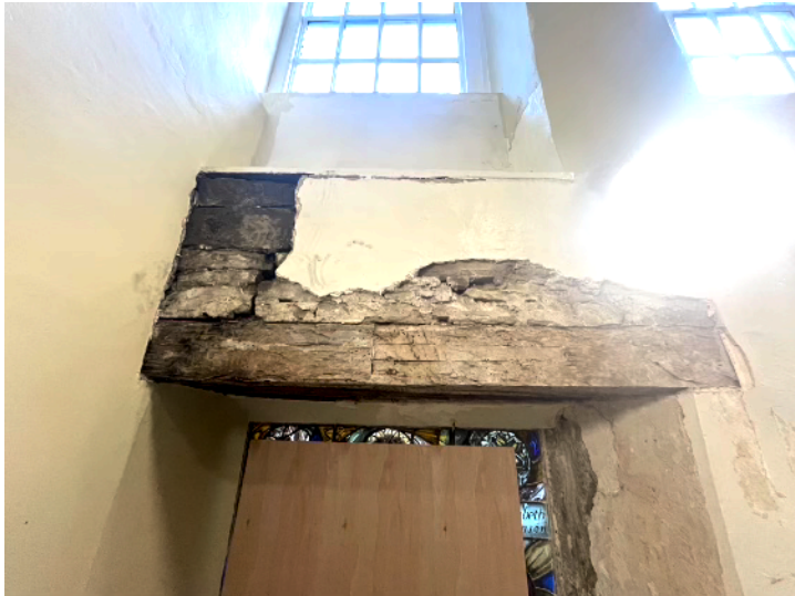
Plaster removed showing past water ingress and lintels.
