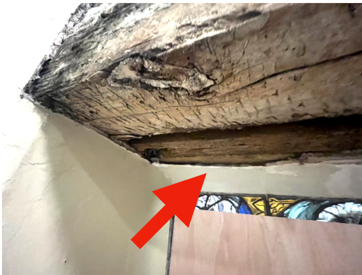
Decayed end of inner lintel.
