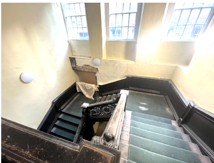
Location on stair makes propping difficult
