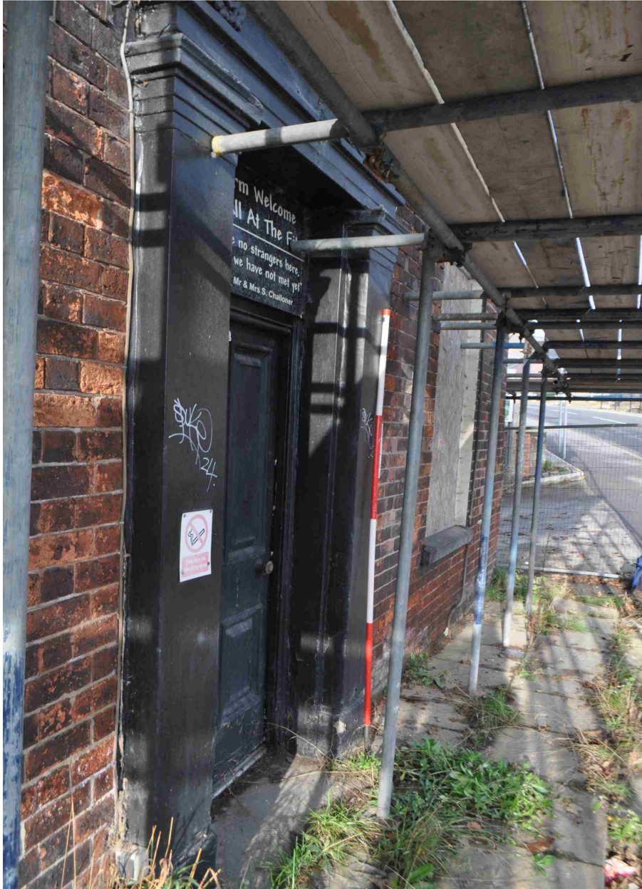
Figure 26: Photo 19. Door, frame and architrave.
