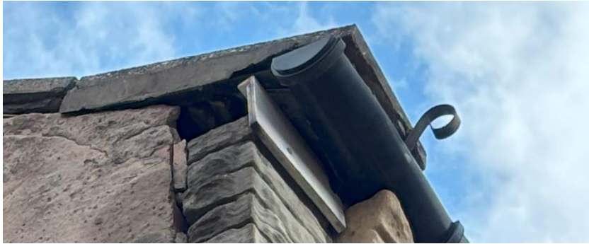
Figure 8 Showing large gap in southwestern corner.
