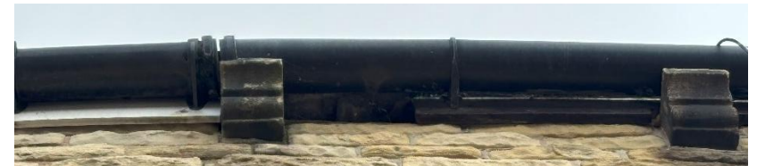
Figure 7 Showing gap between wall top and soffit box.
