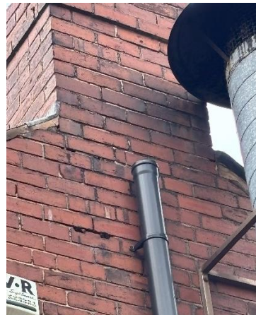
Figure 5 Showing gap in wall.
