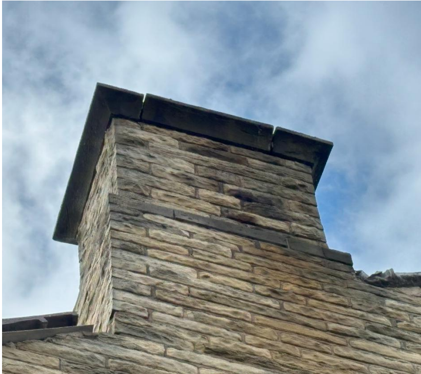
Figure 13 Showing gap between brick and stones on chimney.
