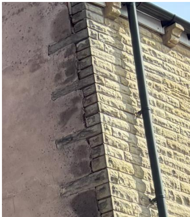
Figure 4 Showing gaps in wall.
