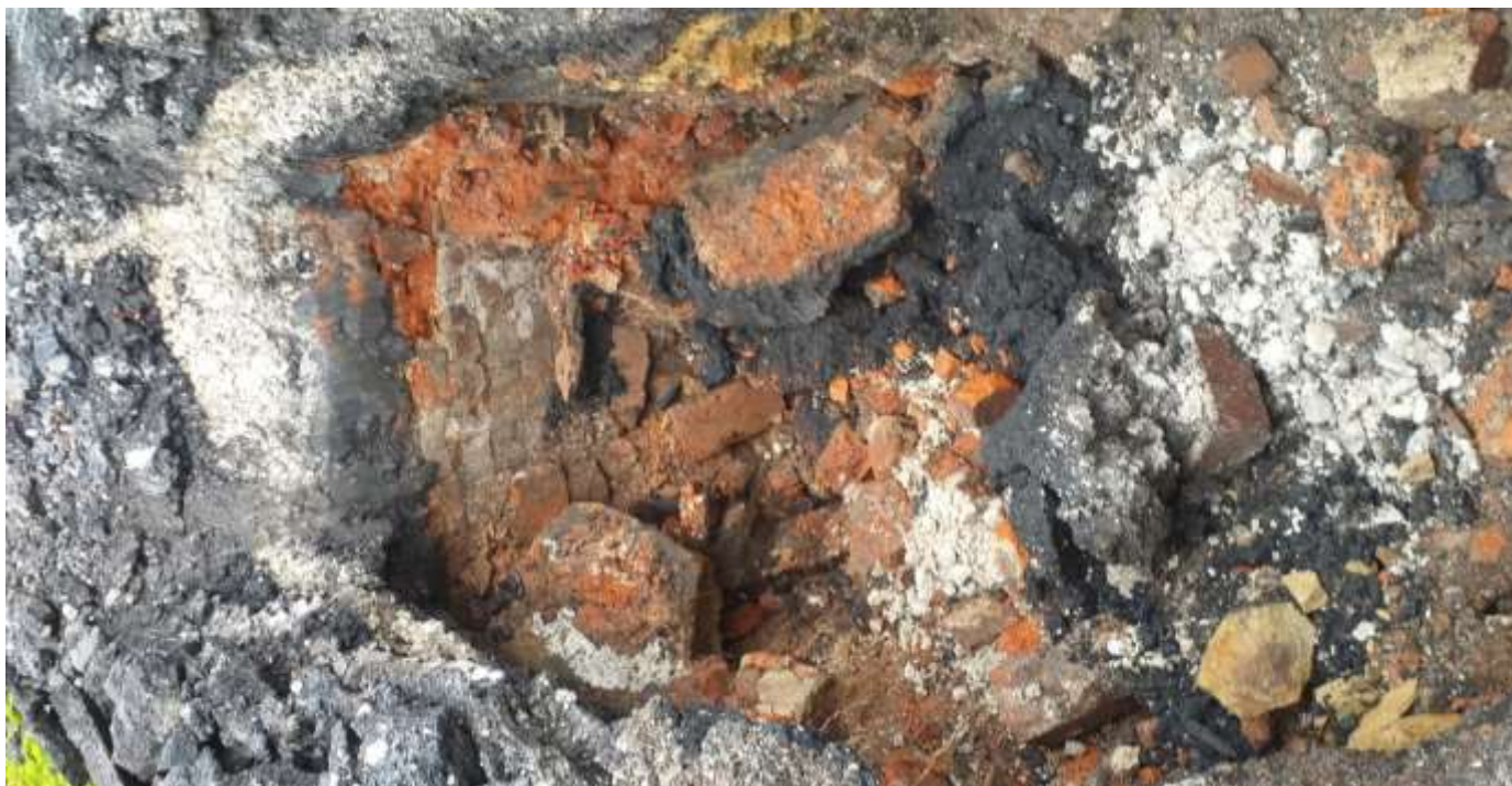
Photo 3: TP3 brick wall obstruction encountered.
