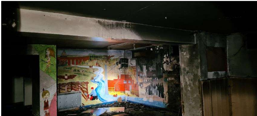
Plate 6. Fire damage on the ground floor
