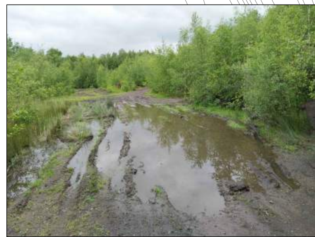
10. Standing water within southern site area.
