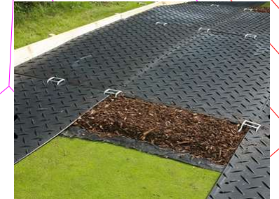
Figure 3: Example of Temporary Ground Protection Boards (GroundGuards) with membrane and woodchip layer:
