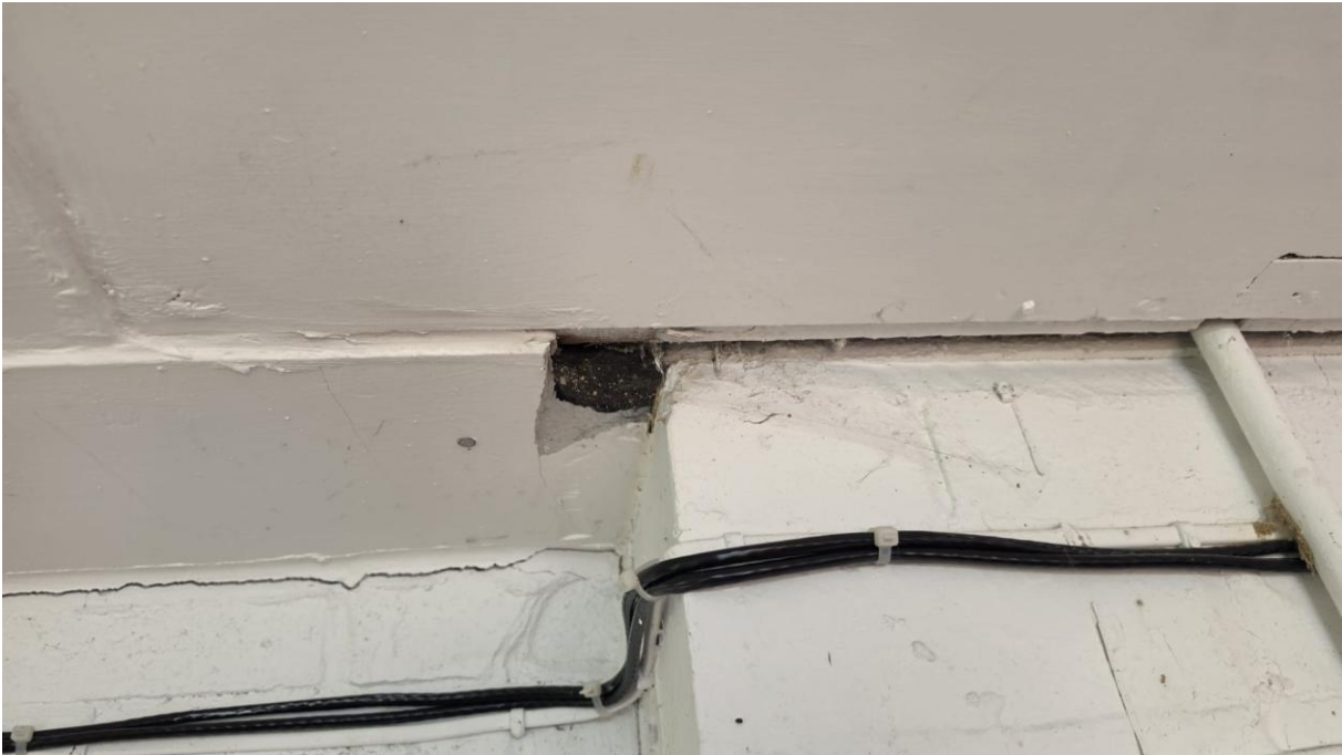
Photograph 7: View of gap in barge boards
