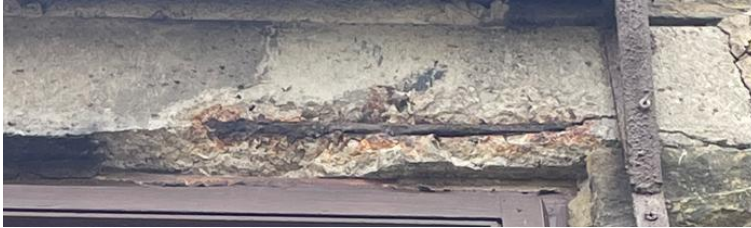
Bedroom window lintel concrete perishing to northerly elevation.
