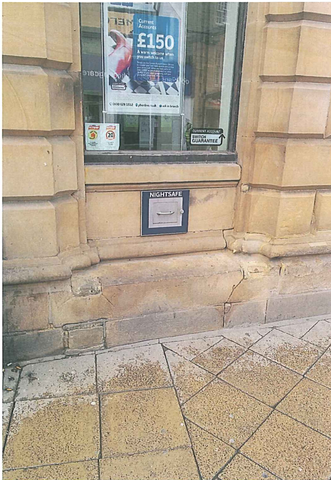
17) WINDOW SILL AT NIGHTSAFE LOCATION
