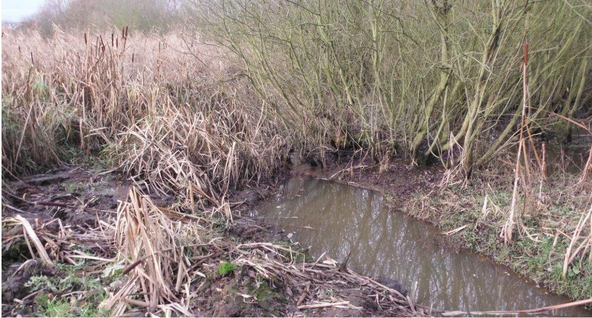
Figure 2-7: Humped Section of Outfall Drain
