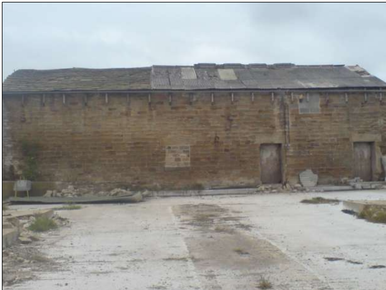
Photo 5: Concrete slab behind milking parlour
