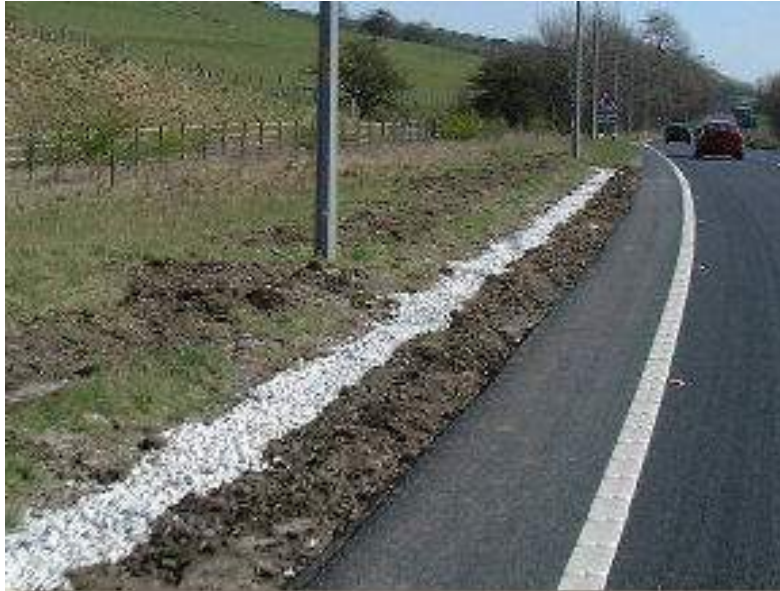
Photo showing edge of carriageway filter strip
