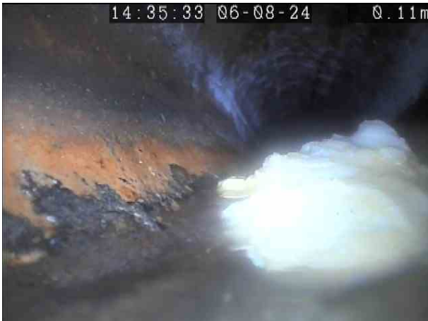
MH9X_b61292d1-0c30-4b2b-b659-c26eacf2a2cb_20240812_121118_358.jpg, 00:00:10, 0.11 m Attached deposits, fouling from 04 o'clock to 08 o'clock, 30% cross-sectional area loss
