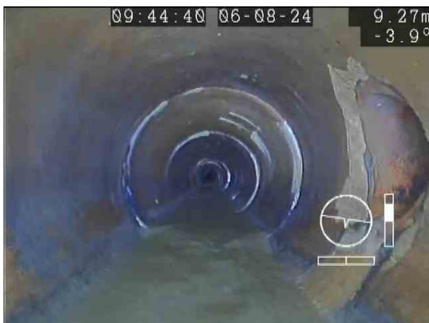
MH2X_cc252805-bd3a-4993-b611-59dcfd49c579_20240812_111721_045.jpg, 00:00:48, 9.27 m Connection other than junction at 03 o'clock, 150mm dia
