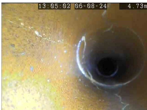
MH4X_6bb3e22b-fa39-4978-ac21-88070a5b0208_20240812_120351_013.jpg, 00:00:28, 4.73 m Cracks, multiple from 12 o'clock to 12 o'clock
