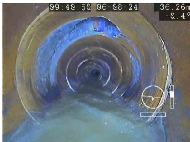
MH1X_0d9a47b8-c179-421c-9966-5658da730b5a_20240812_111402_502.jpg, 00:02:41, 36.26 m Connection other than junction at 12 o'clock, 100mm dia
