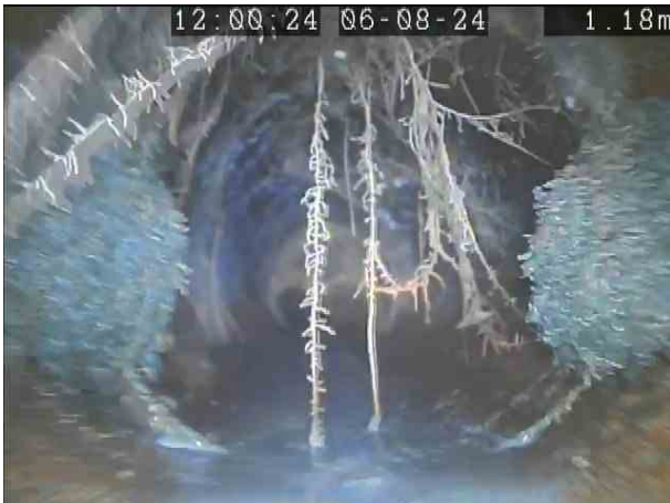
UpstreamX_b0335336-3924-4b33-a2be-40099bb87b09_20240812_114204_616.jpg, 00:00:15, 1.18 m Roots, mass at joint, 25% cross-sectional area loss
