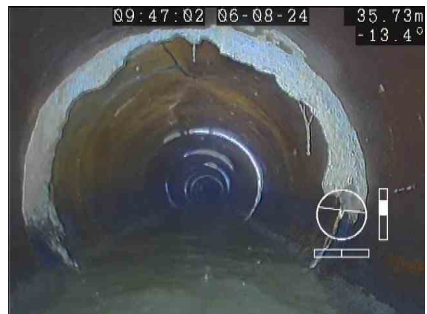
MH2X_dee560cd-5f12-4c64-963a-88c51db298de_20240812_111948_233.jpg, 00:03:10, 35.73 m Crack, longitudinal at 12 o'clock
