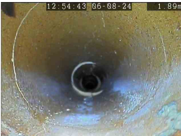
UpstreamX_56508c19-a7f9-4108-8dab-9e6aa03b9b98_20240812_114906_832.jpg, 00:00:40, 1.89 m Crack, circumferential from 12 o'clock to 12 o'clock
