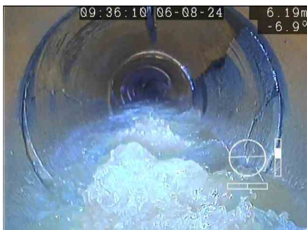
MH1X_57331753-2901-490a-b26d-40df08841c2e_20240812_111305_771.jpg, 00:00:50, 6.19 m Fractures, multiple from 12 o'clock to 12 o'clock
