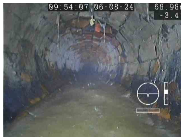
MH2X_17d61786-185a-4e1b-82ea-5b547061bb71_20240812_112324_575.jpg, 00:06:47, 68.98 m Connection other than junction at 12 o'clock, 150mm dia
