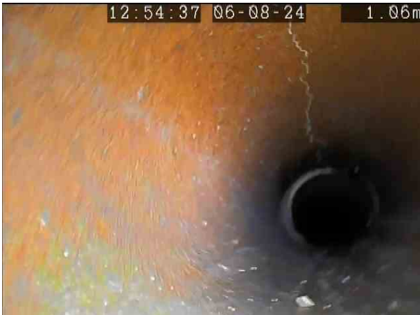
UpstreamX_2073ff9d-1059-4bdf-8054-2b143b36b8bf_20240812_114833_120.jpg, 00:00:34, 1.06 m Crack, longitudinal at 12 o'clock
