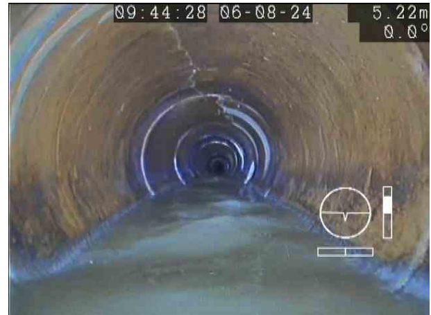
MH2X_6db244d5-3ff5-431f-bfec-cfd338009be2_20240812_111652_207.jpg, 00:00:35, 5.22 m Crack, longitudinal at 11 o'clock, start
