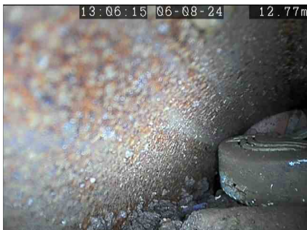
MH4X_dce3b7e3-68ce-42c4-944b-711f0315f6dd_20240812_120454_527.jpg, 00:01:10, 12.65 m Settled deposits, coarse, 95% cross-sectional area loss
