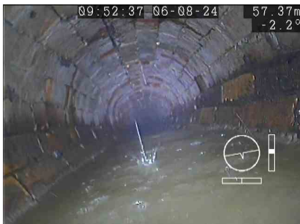
MH2X_5635edc3-1272-4f0a-9816-837d2ba72dcf_20240812_112134_435.jpg, 00:05:16, 57.37 m Infiltration, dripping from 10 o'clock to 02 o'clock, start
