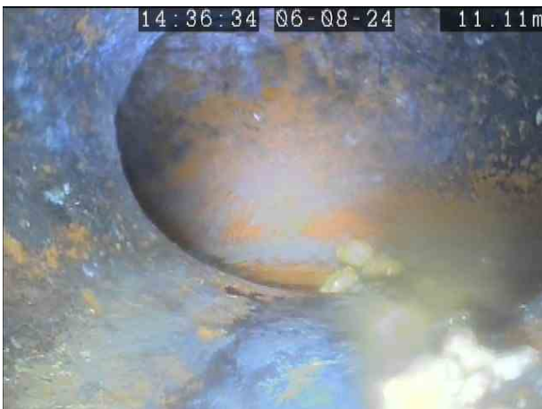
MH9X_b4188a44-f55b-49ee-b505-0b5ae8c3b84a_20240812_121212_354.jpg, 00:01:04, 11.11 m Line deviates left, INTO JUNCTION
