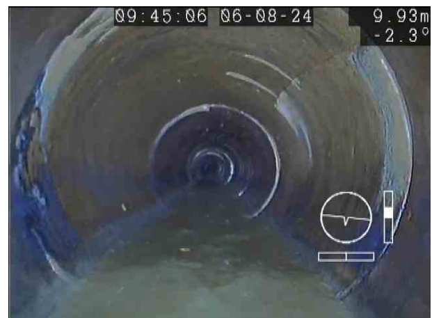
MH2X_8b485754-31ee-4d55-9e34-2c7c51316338_20240812_111744_612.jpg, 00:01:13, 9.93 m Crack, longitudinal at 02 o'clock
