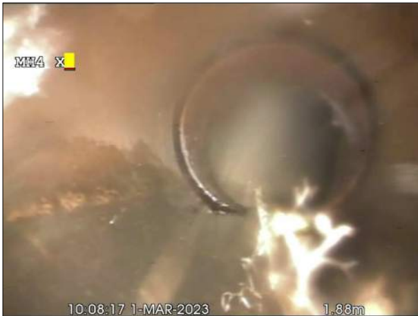
Photo: 42_4a, 00:00:00 1.9m, Joint displaced. Medium
