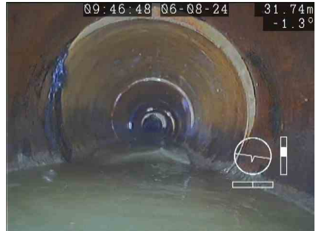
MH2X_d2c1b144-da18-423f-8fe2-9c940f5444cc_20240812_111859_743.jpg, 00:02:55, 31.74 m Joint displaced, medium
