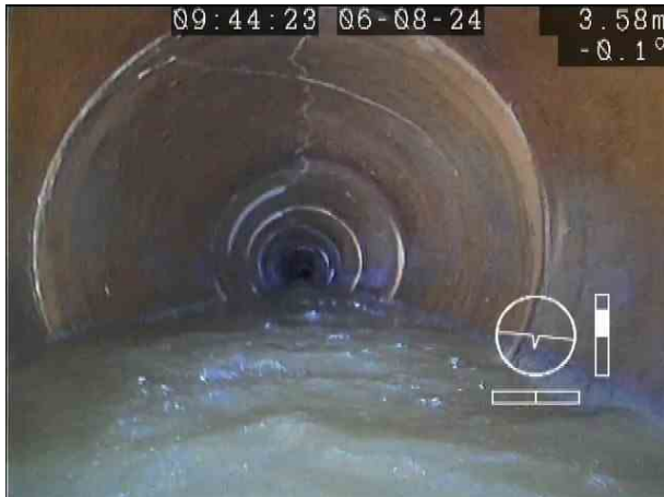
MH2X_343fe477-d113-4899-a973-9e4abd930d52_20240812_111631_725.jpg, 00:00:30, 3.58 m Cracks, multiple from 10 o'clock to 03 o'clock
