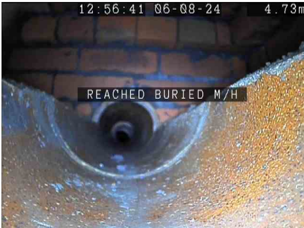
UpstreamX_305cf42b-dc3d-4801-b555-6358f9682f41_20240812_115001_507.jpg, 00:01:34, 4.73 m General photograph taken at this point, buried manhole
