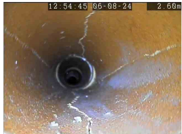
UpstreamX_342c907d-01b5-48cb-a028-132170947893_20240812_114927_787.jpg, 00:00:42, 2.60 m Cracks, multiple from 12 o'clock to 12 o'clock
