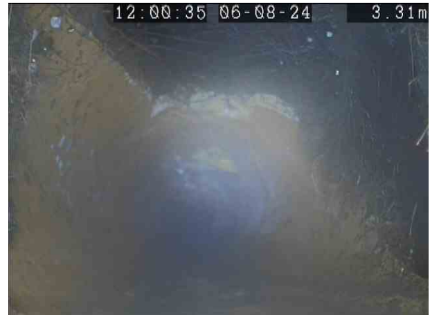
UpstreamX_0cc2a8b9-c6fe-4dc4-8f75-75a0937ea0fd_20240812_114226_042.jpg, 00:00:26, 3.31 m Hole in drain or sewer from 01 o'clock to 05 o'clock
