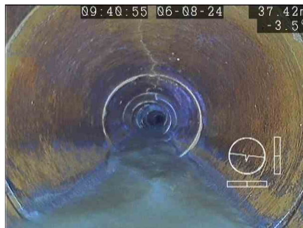
MH1X_cafab7d0-50e5-4003-9632-e5a048611cf2_20240812_111451_058.jpg, 00:02:44, 37.10 m Crack, longitudinal at 12 o'clock, start
