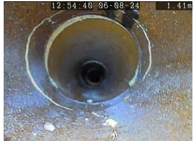
UpstreamX_139ac17c-f647-4501-9898-87e944ac7036_20240812_114850_286.jpg, 00:00:37, 1.41 m Fracture, circumferential from 12 o'clock to 12 o'clock
