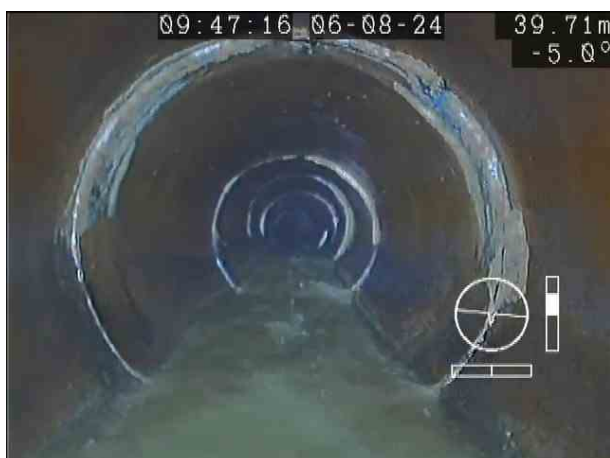
MH2X_c372f123-ab27-44c4-afbf-3fa92f379988_20240812_112019_377.jpg, 00:03:23, 37.91 m Infiltration, dripping at 12 o'clock
