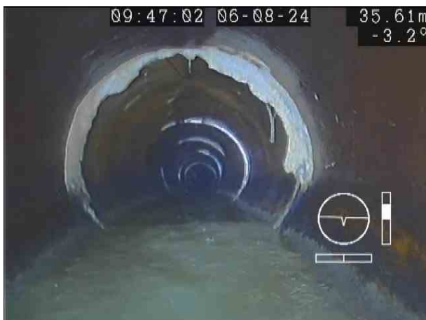
MH2X_ad42cbe7-0a16-4016-9956-fc94c6be4d1a_20240812_111922_830.jpg, 00:03:09, 35.61 m Attached deposits, encrustation at joint from 07 o'clock to 04 o'clock, 10% cross-sectional area loss
