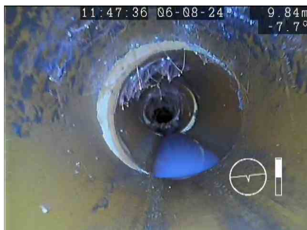
Exc Pipe1X_041e4a96-962b-4fe0-88a0-0faee3dbe9b0_20240812_113726_191.jpg, 00:01:10, 9.84 m Joint displaced, medium
