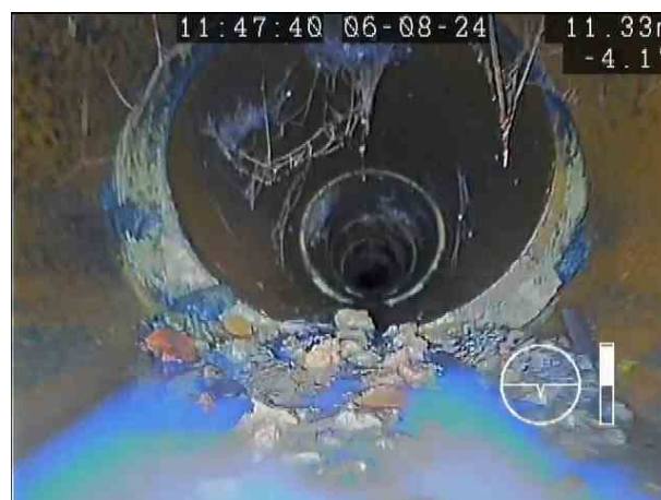
Exc Pipe1X_105ee651-1135-472e-ba40-8f5d479d03a8_20240812_113739_703.jpg, 00:01:14, 11.33 m Joint displaced, medium
