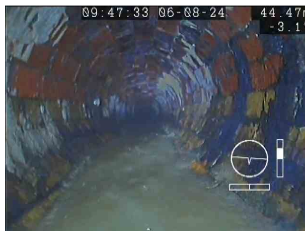
MH2X_ab00335a-4fe4-4e54-8d0e-c2fd4113e1cd_20240812_112037_954.jpg, 00:03:40, 44.47 m Pipe material changes to brick at this point
