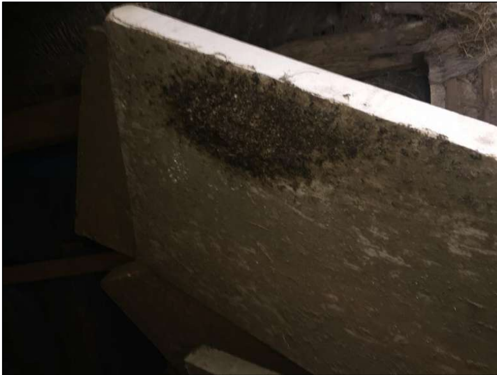
Plate 9: Aggregate of swallow droppings in building 1
