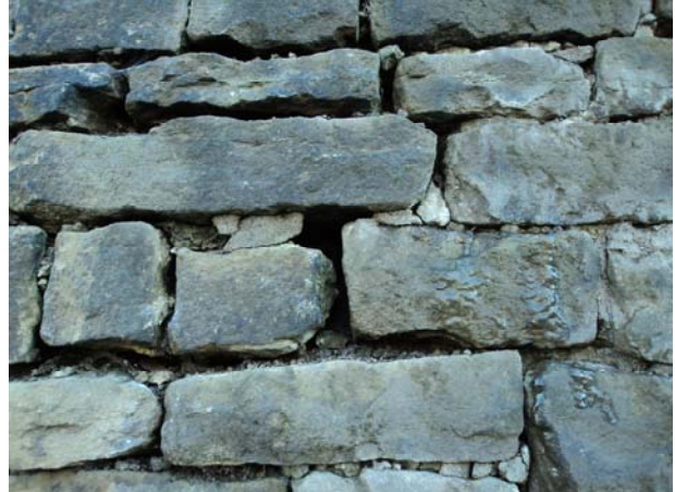
Plate 3.2: Example of missing mortar
