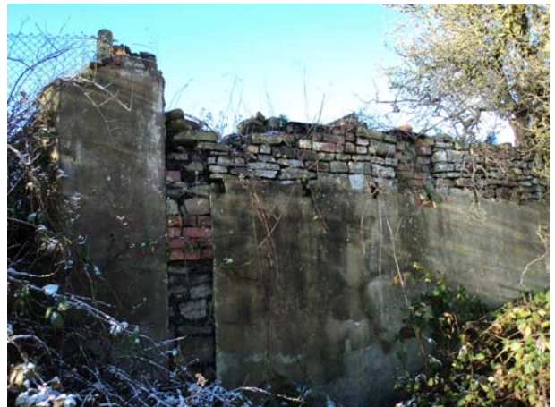
Plate 3.4: Dilapidated section of brick wall
