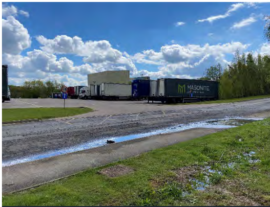
Photo 7: View looking east towards lorry park – note water issuing at surface on western plot
