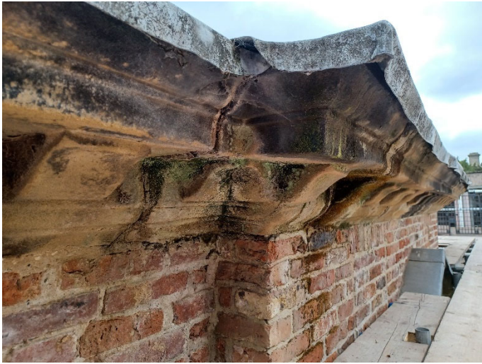
Water staining and vegetation growth on the west elevation
