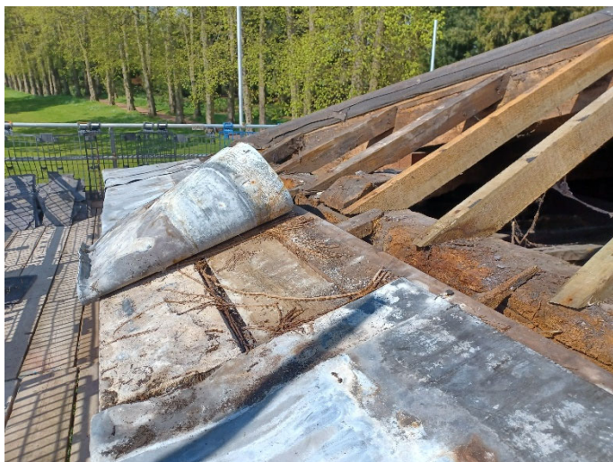
Simple lap detail and underside corrosion on the apron flashing to the stone cornice
