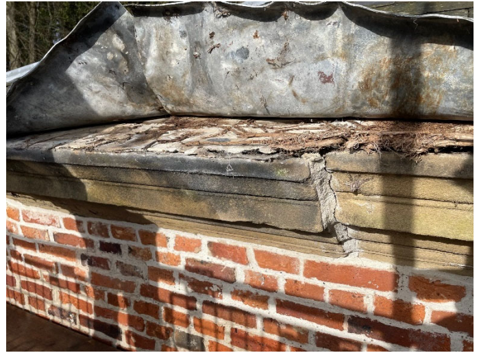
Displaced cornice stone and dead ivy growth beneath the lead apron
