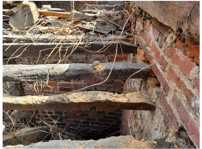
Ceiling joists have lost their connection to the wall on the south elevation in G1
