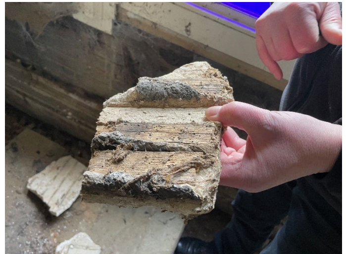
Laths still attached to a section of plaster fallen. Small insect flight holes present and the laths are brittle and friable.
