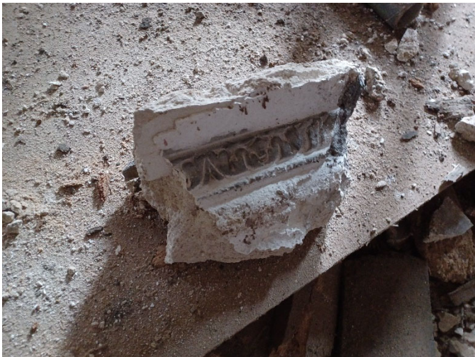
Section of cornice that has fallen away in G1
