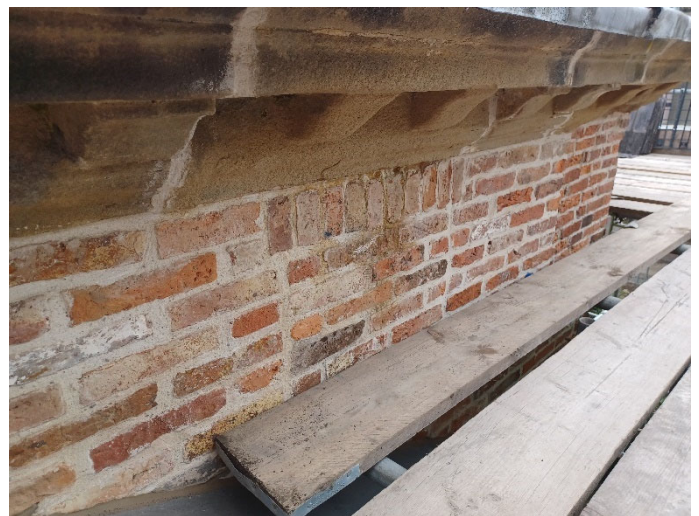
Loss of detail observed on the west elevation
