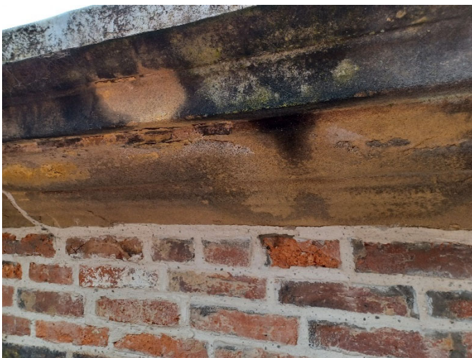
Ongoing delamination to the cornice on the north elevation
