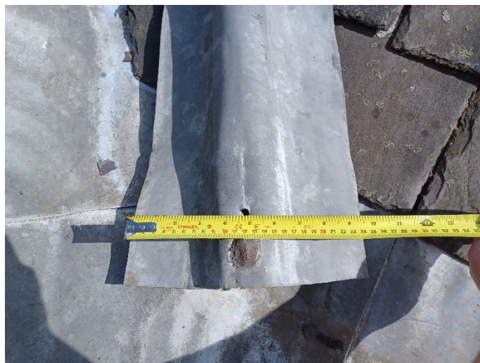
Extent of cover from hip flashings together with tear from mechanical fixing through the top of the sheet
