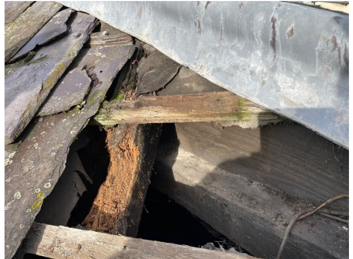
Decayed rafter and roof laths and perished underfelt to southeast corner
