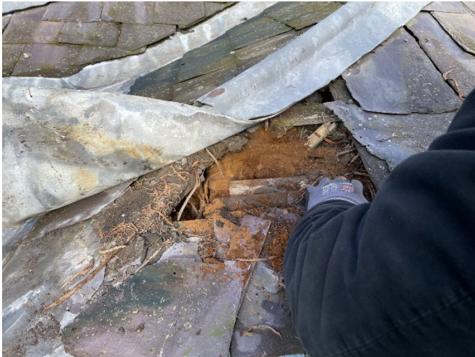
Severely decayed wall plate ends to the southwest corner
