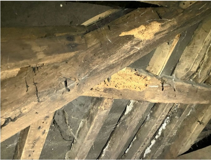
Insect activity and water staining to the hip rafter and purlin on the northwest corner
