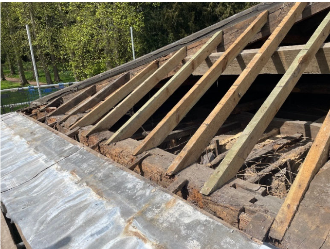
Replacement rafters and purlin provided to the west end of the south elevation and detail of
