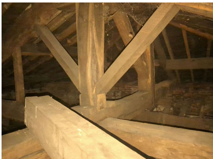
General view from northwest corner of roof void looking diagonally across at the back of the east and south facing roof pitches prior to opening up
