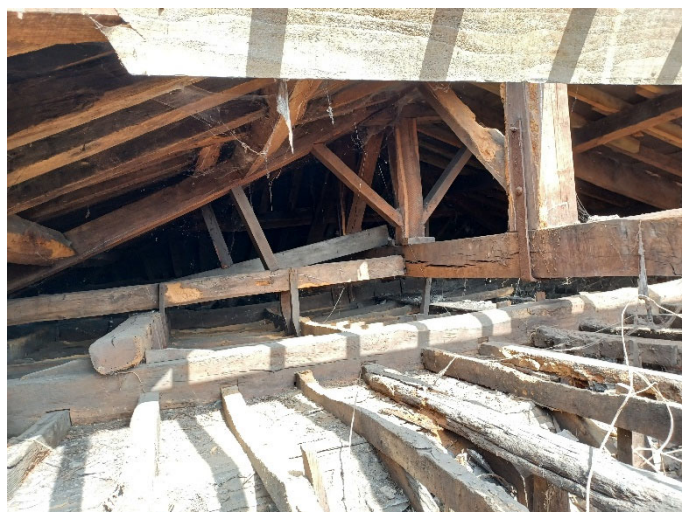
View of roof structure through the south roof slope following removal of roof coverings
