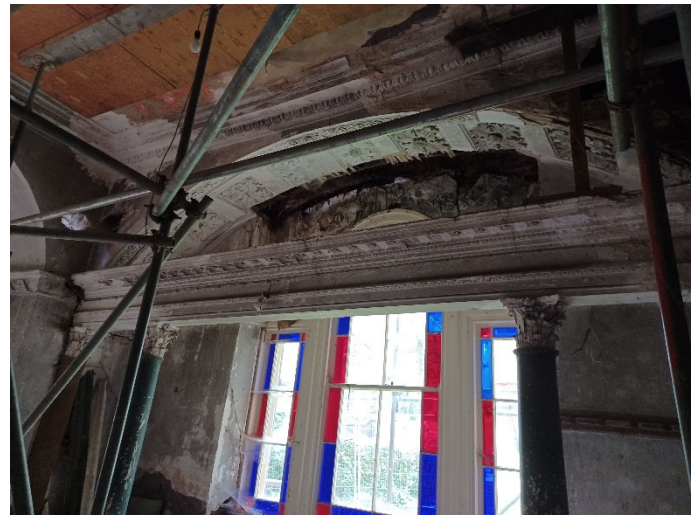
Central section of ceiling lost in the bay window
