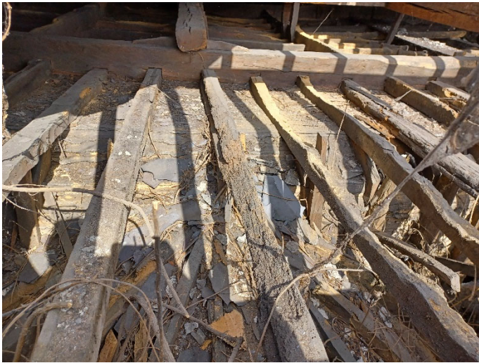
Significant cross sectional loss to the ceiling joists above G1
