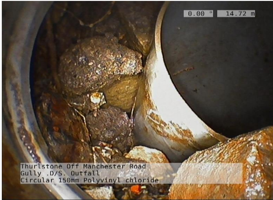
Gully-DOutfall-5-29960.jpg, 00:01:10, 14.72 m Joint displaced, large
