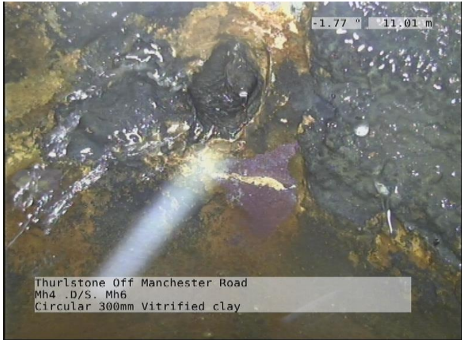
Mh4-DMh6-3-52642.jpg, 00:00:59, 11.01 m Hole in drain or sewer at joint at 12 o'clock
