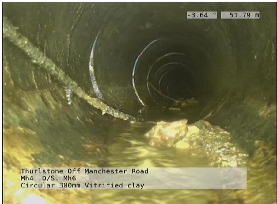
Mh4-DMh6-4-19649.jpg, 00:03:19, 51.79 m Roots, tap at joint
