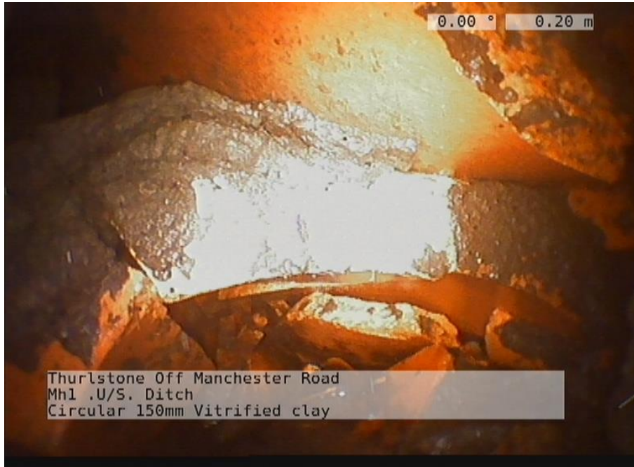
Mh1-UDitch-1-8473.jpg, 00:00:15, 0.20 m Collapsed drain or sewer
