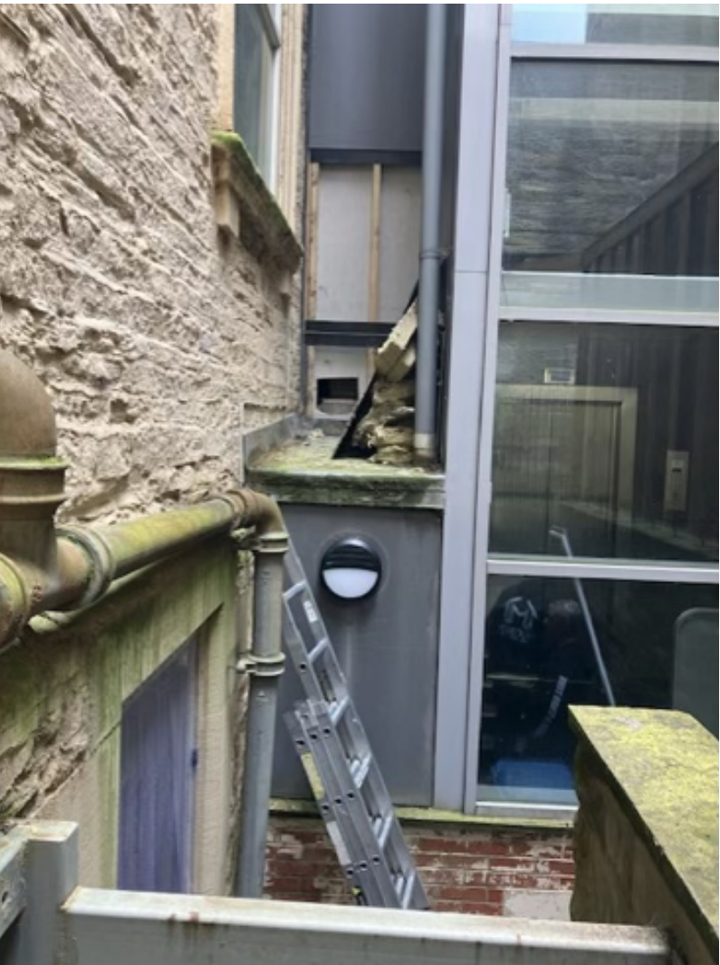
Existing fan housing with exhaust housing and duct opened behind.
