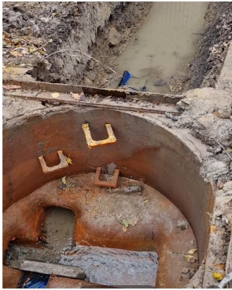
Figure 16 Chamber 3 with blue field drain visible at the bottom of the picture
