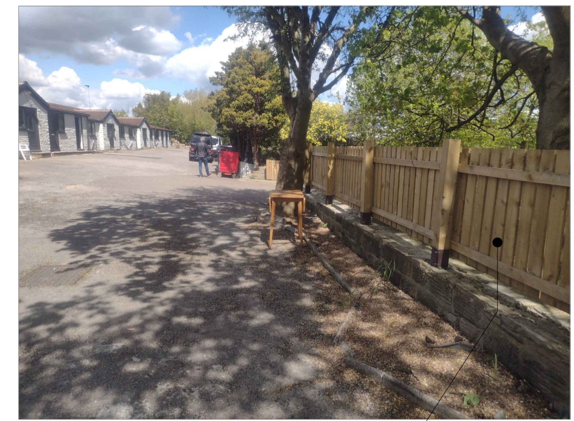
Photo 2: Remove existing timber fence posts and panels. Retain existing steel pockets and ensure security fixed to wall. Provide new timber posts and panels to create new fence height of 1.8m above ground level.
