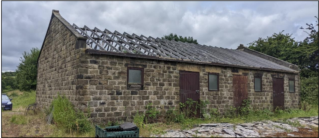
Plate 3. Evidence of bat roost recorded from south elevation of former stables
