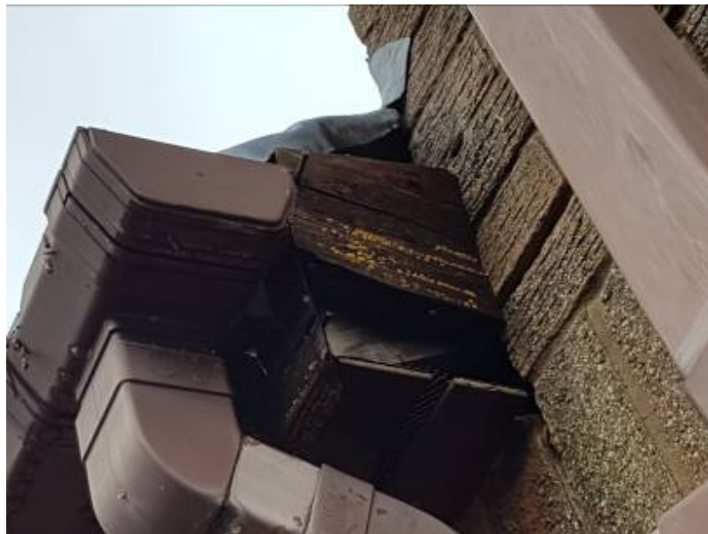
Photograph 1a Minor gap at soffit board
