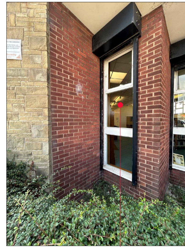
Photo 17 Existing external view of windows ExWLL01 to 04. Windows to be removed and replaced with new - refer to window schedule for proposed pattern. Existing shutters externally to be retained.
