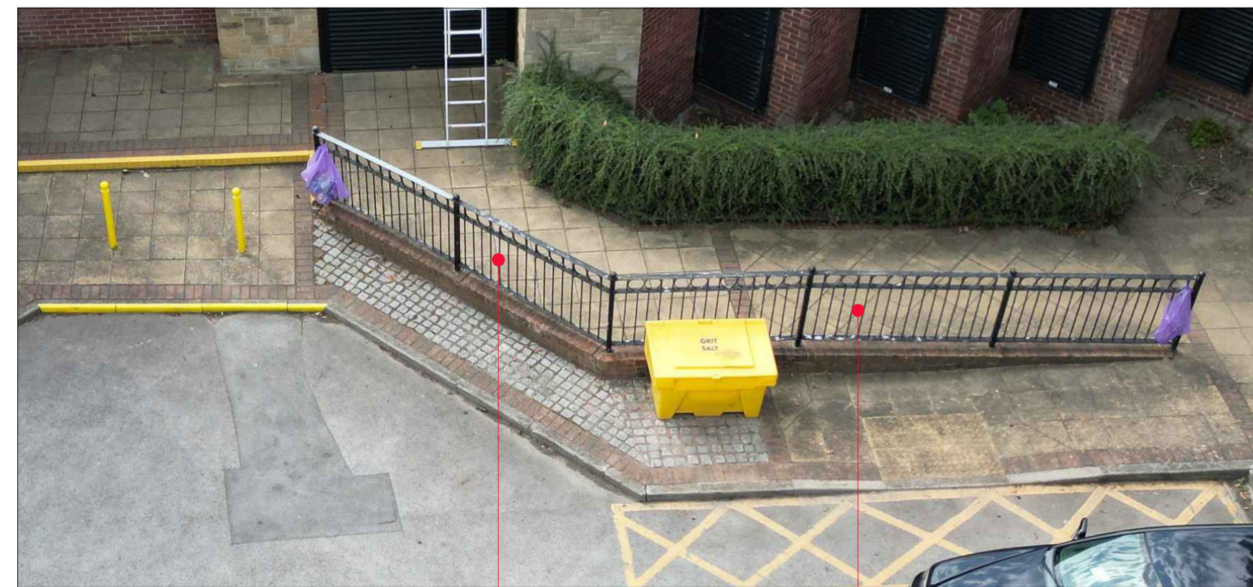
Photo 21 Existing balustrade to be prepared to receive new suitable paint decoration finish. Repair / replace all spalled / damaged brickwork to low wall.
