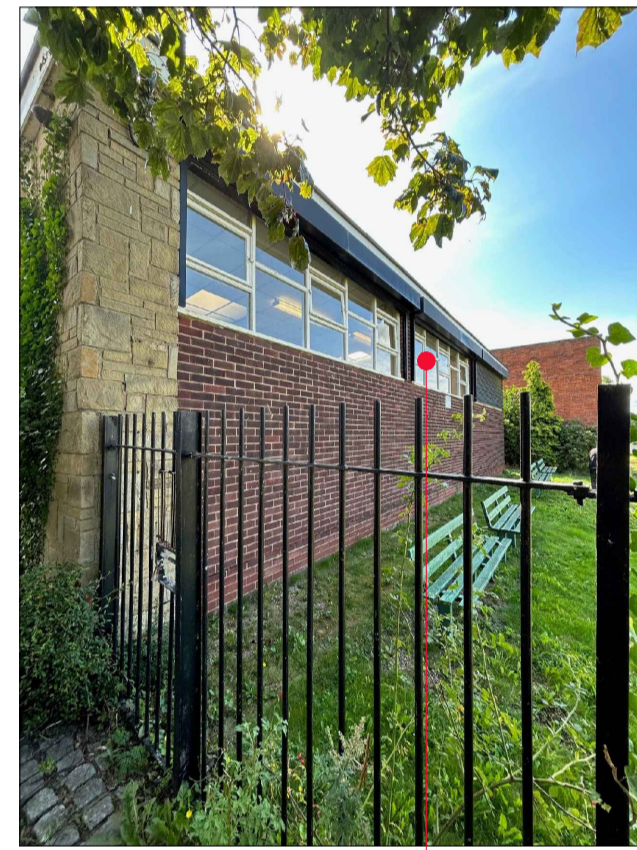
Photo 18 Existing external view of windows ExWML05, 06 & 07. Windows to be removed and replaced with new - refer to window schedule for proposed pattern. Existing shutters externally to be retained.
