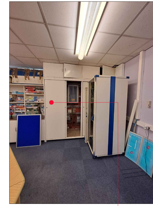
Photo 15 Existing full height cupboard to enclose electrical switch gear to be removed. Construct new fire rated partition & door-set.
