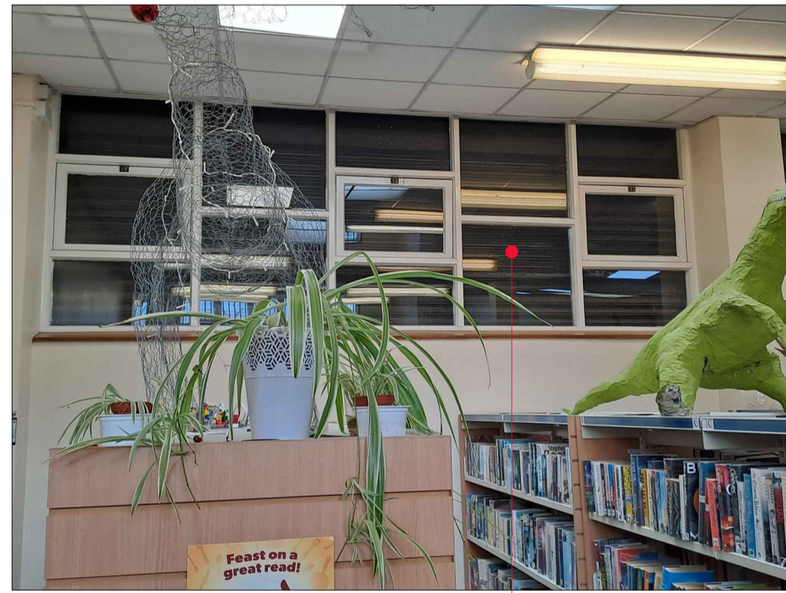
Photo 16 Existing windows ExWML05, 06 & 07 to be removed and replaced with new to match existing fenestration pattern. Existing shutters externally to be retained.
