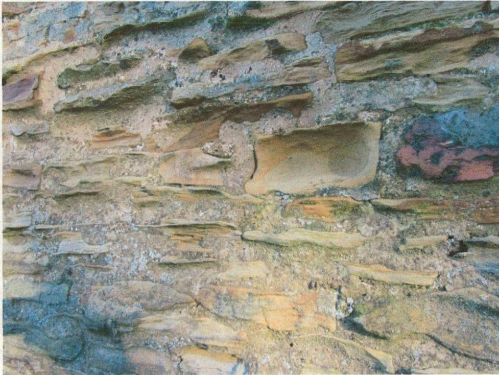
Photo 25 – Enlarged view. Note – severe weathering of poor quality stone.
