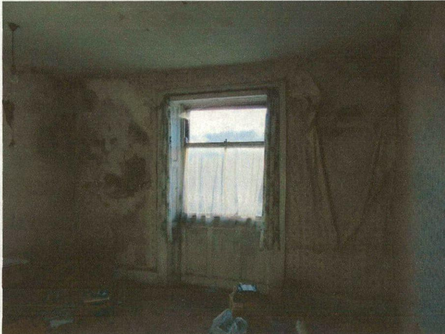
Photo 28 – Internal view of first floor front wall to No 323. Severe water ingress from gutters.
