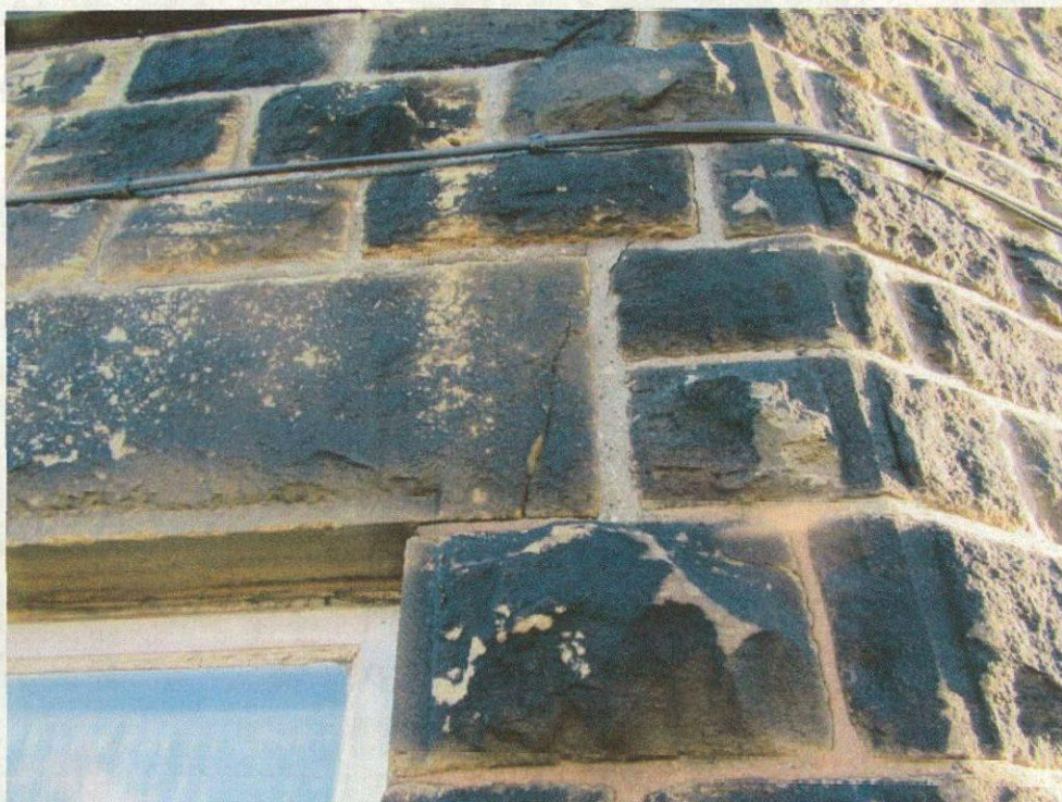
Photo 22 – Failure of lintel bearing.
