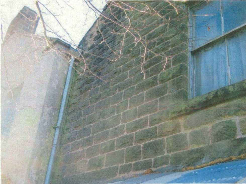
Photo 9 – Crack at junction of rendered front and rear stone work behind rainwater pipe, as the front is moving out more than the rear. Note – poor valley gutter outlet.
