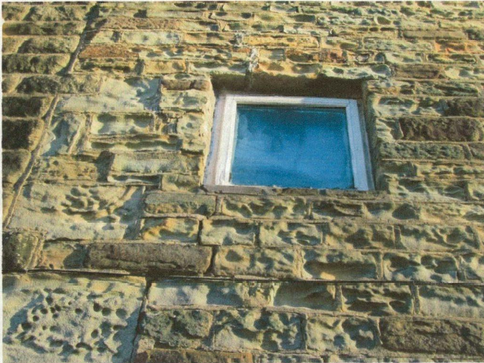
Photo 15 – Cracking between two gable ends below first floor window. Note – lack of lintel over window.
