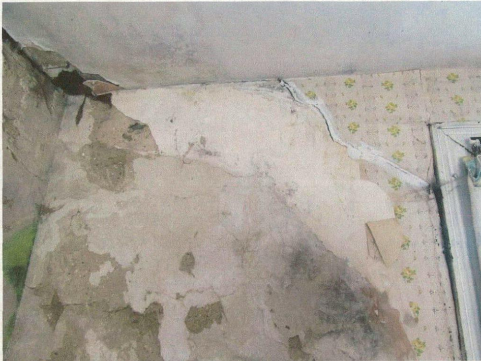
Photo 29 – Settlement cracking to upper right corner, as the gable panel settles.
