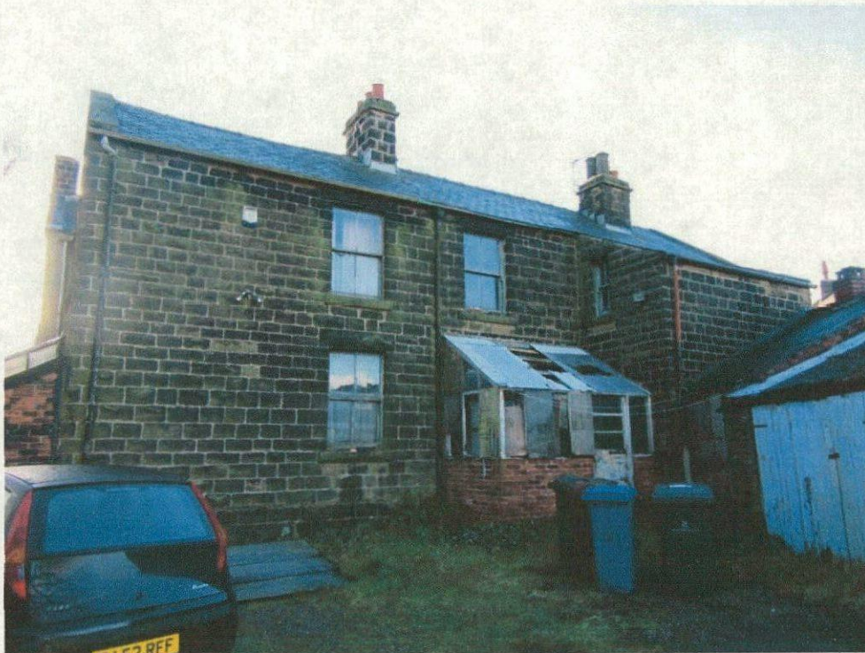
Photo 10 – General view of the rear of No 321 (centre) and No 323 (left of view) and No 2 Haigh Lane. Monopitch to the right of view includes ancillary buildings. Porch to the rear of No 321 is severely dilapidated.
