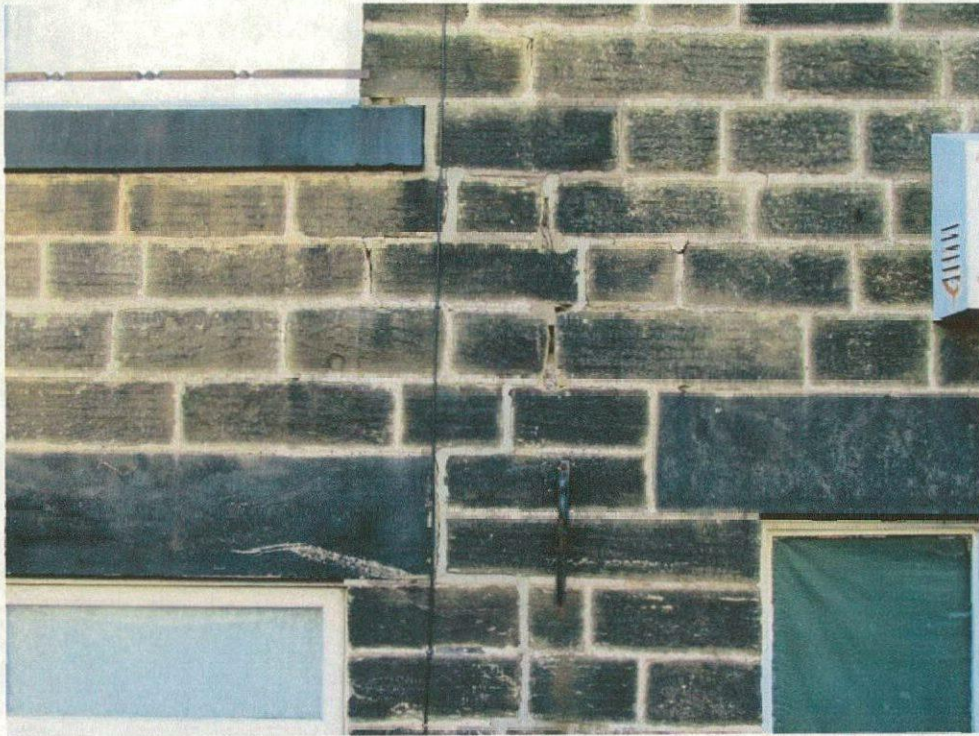
Photo 3 – Vertical cracking between ground floor lintels and first floor sill.
