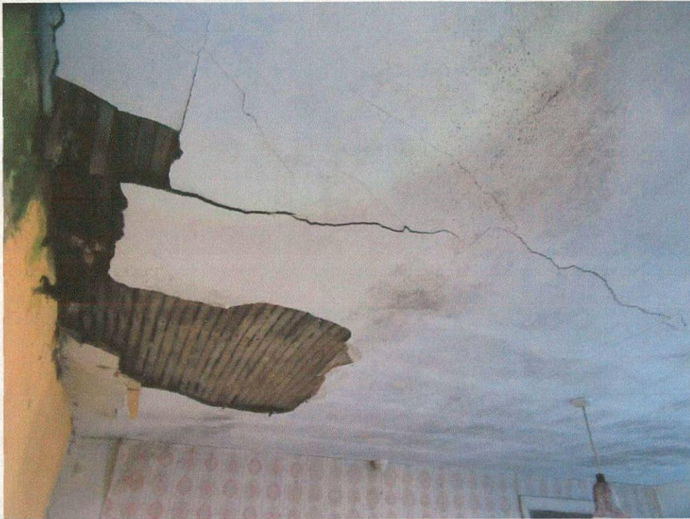
Photo 37 – Water ingress at valley line with rotten timbers present.
