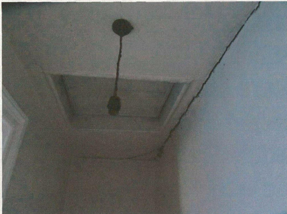
Photo 40 – Severe internal settlement of No 2 Haigh Lane/ No 319.
