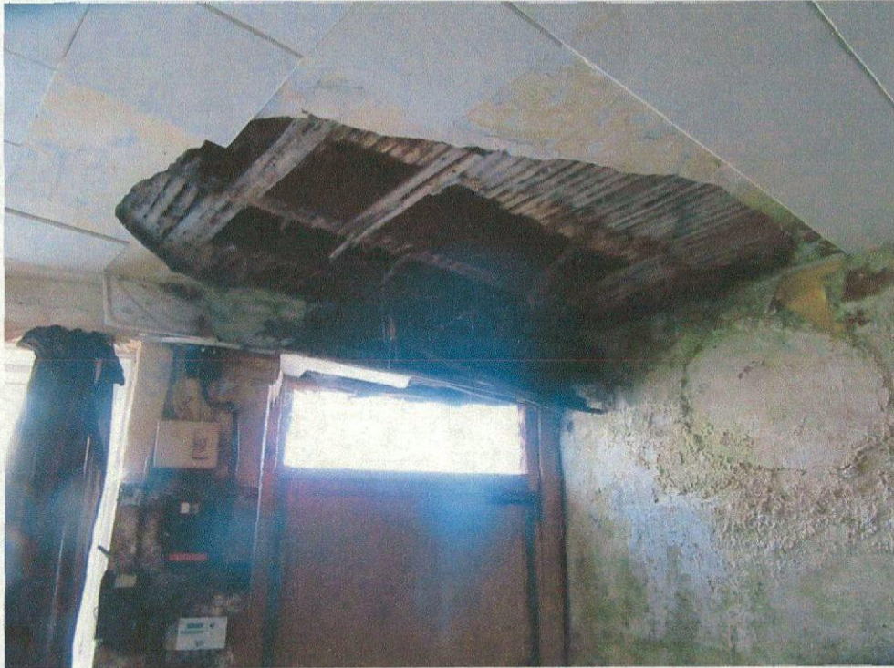
Photo 41 – Rear left hand gable of 2 Haigh Lane. Severe water ingress – rear left corner.
