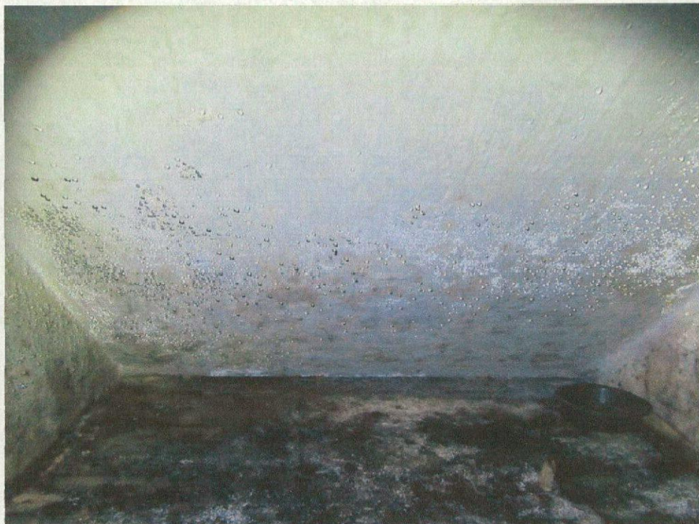
Photo 42 – Condensation from water in the cellars at No 319. It is believed there may be a well beneath the property.
