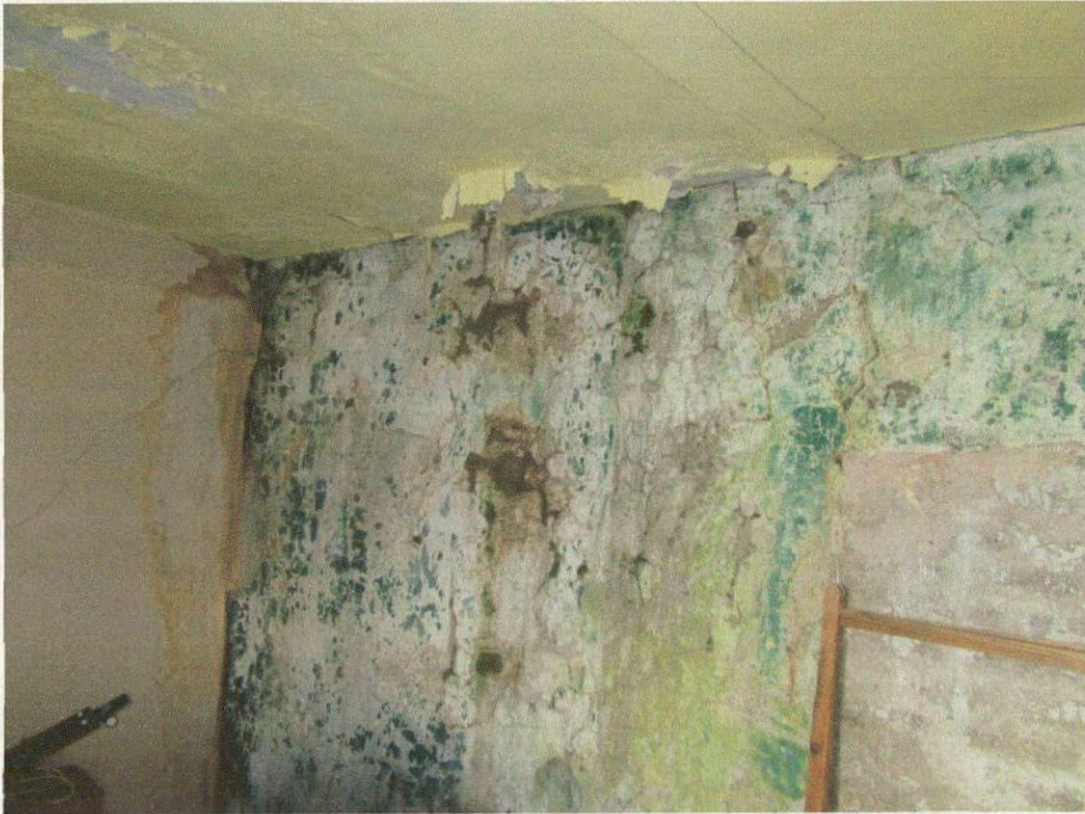
Photo 33 – Water damage on valley line of No 321.
