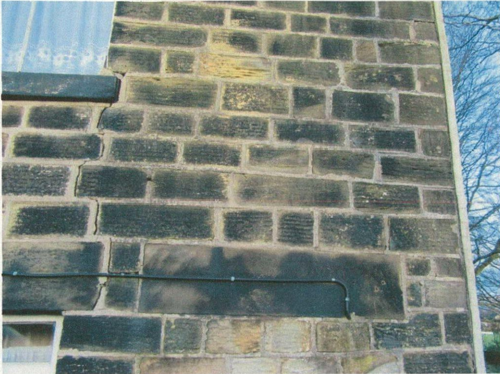
Photo 5 – Right hand gable and end of front wall has severe settlement to No 323. Note – 50mm settlement of old lintel over walled up original doorway and severe crack between lintel and first floor sill stone.
