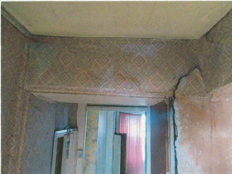
Photo 35 – Internal view looking from the front of No 323, through a doorway towards the rear. Note – severe settlement to right hand of the lintel members as the wall is settling.
