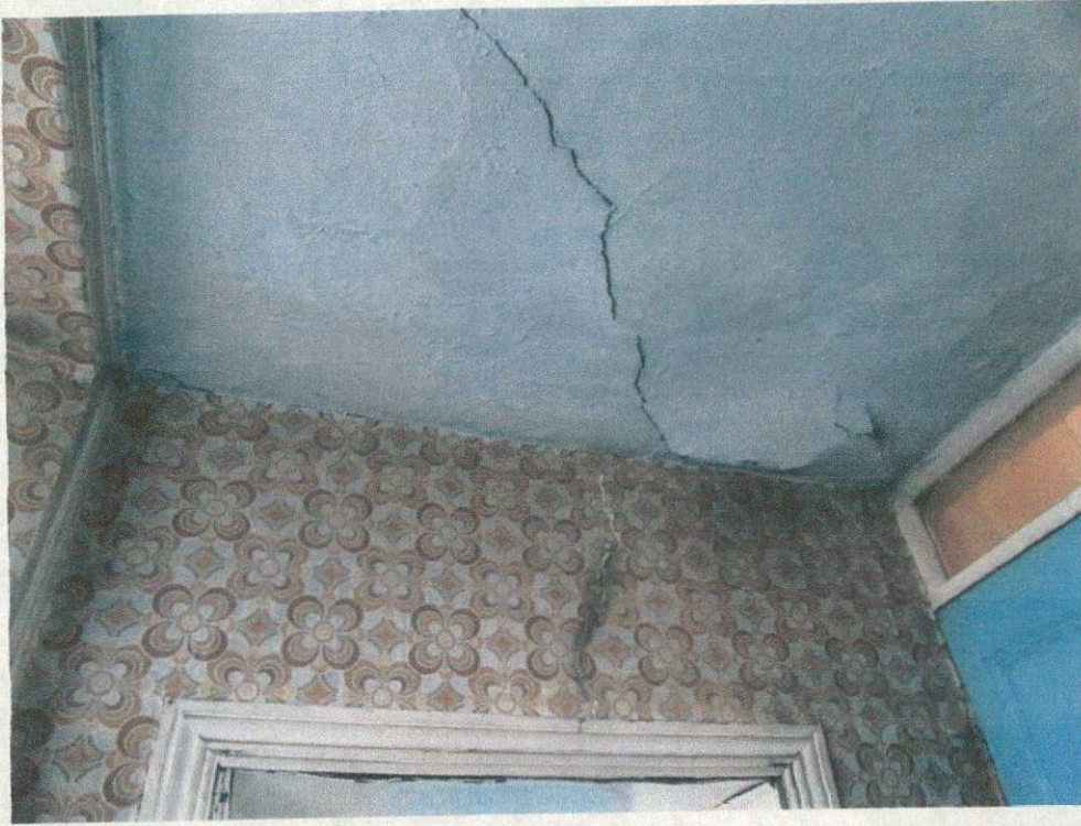
Photo 45 – Settlement of internal wall at No 323 and cracking of ceiling.
