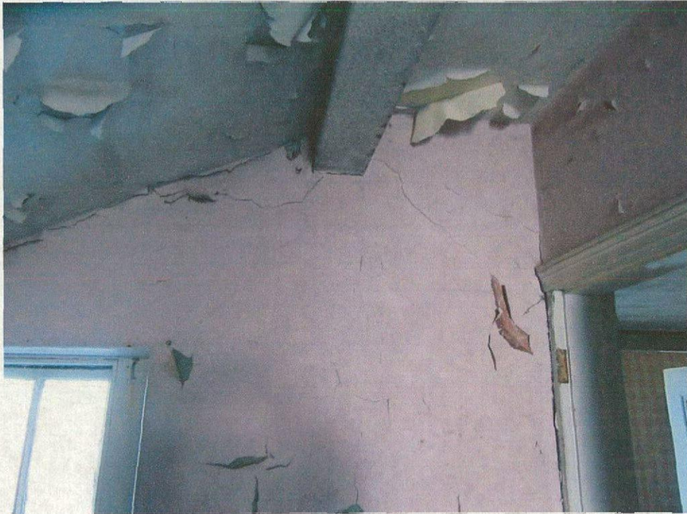
Photo 39 – Settlement to right hand gable of No 2 Haigh Lane.
