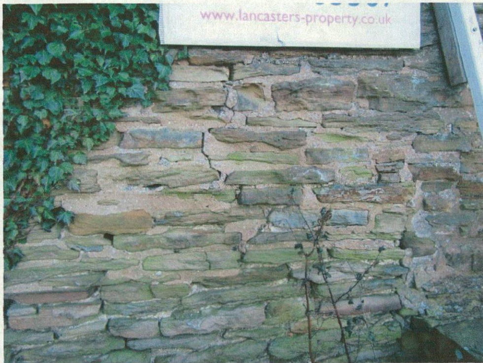
Photo 13 – Movement cracks to gable of outbuilding.
