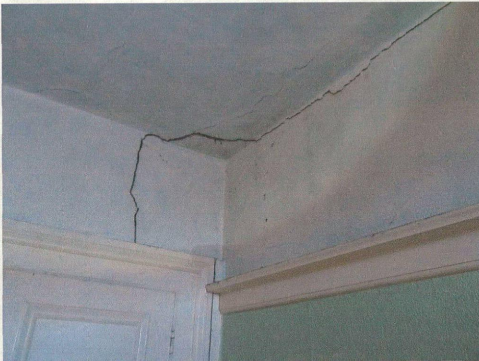
Photo 44 – Internal cracking due to settlement of gable.
