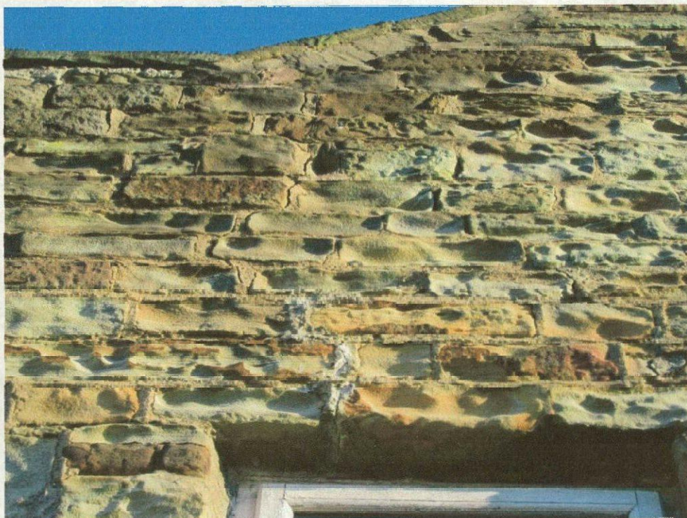
Photo 16 – Vertical crack above same window.
