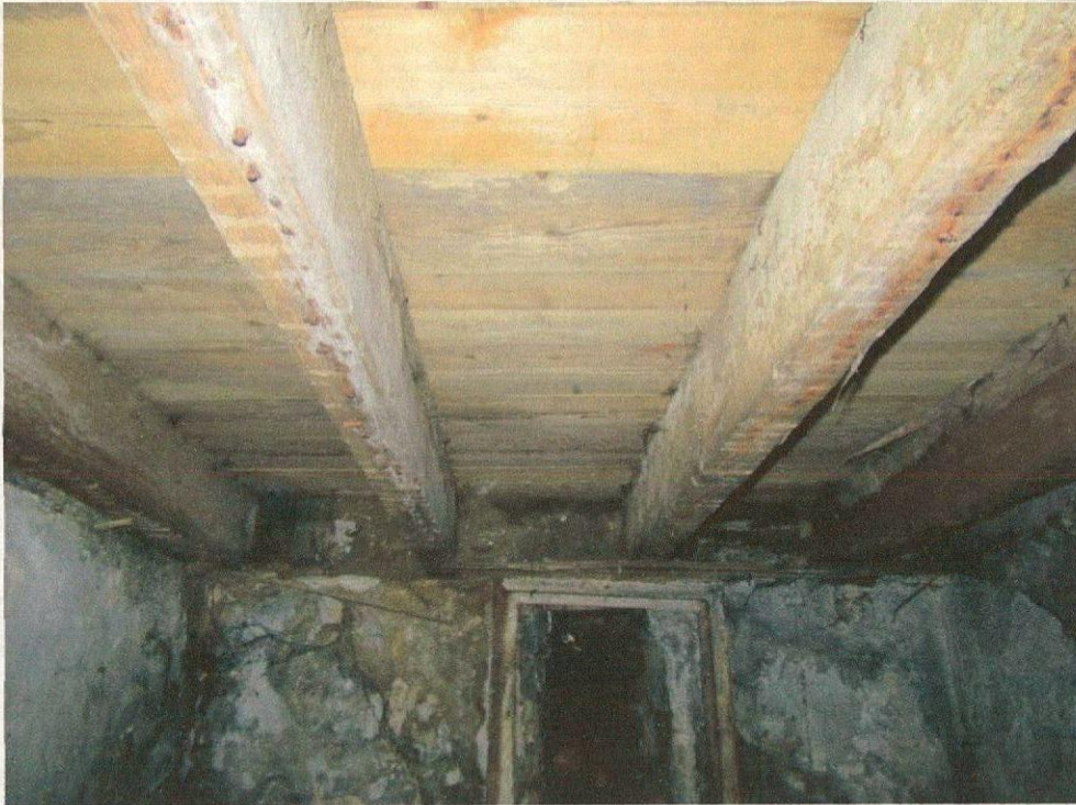
Phot 47 – Cracking to stone wall and rotten floor joists.
