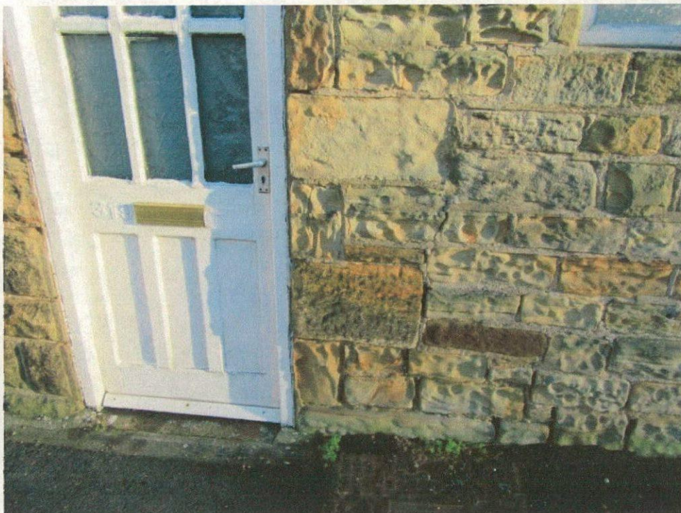
Photo 20 – Cracking to gable of No 319.
