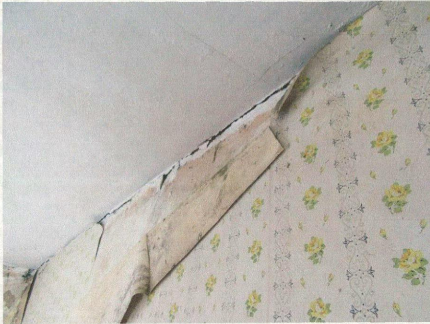
Photo 31 – Further internal settlement to No 323.
