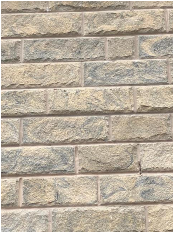
Photo showing the stone sample is to be used on the walling. The stone is Cromwell pitched- weathered walling stone random sizes 300/440 x 100 x 140 (see brochure attached).
