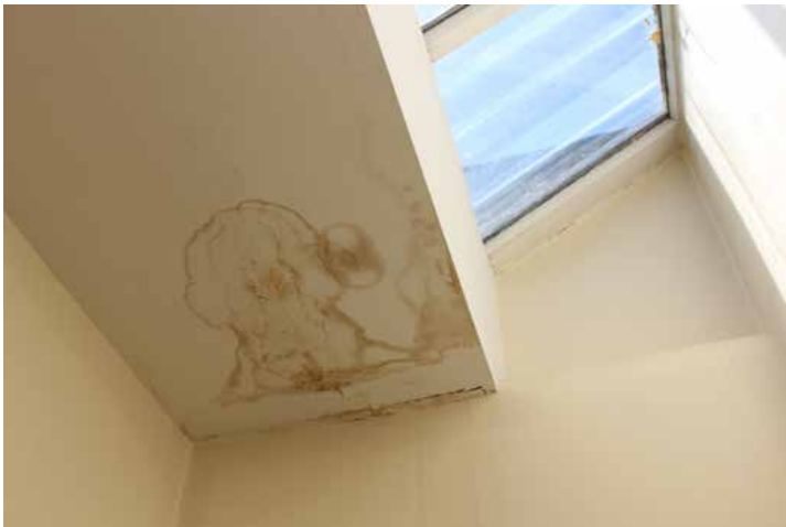
Building 13, water ingress staining below rooflights
