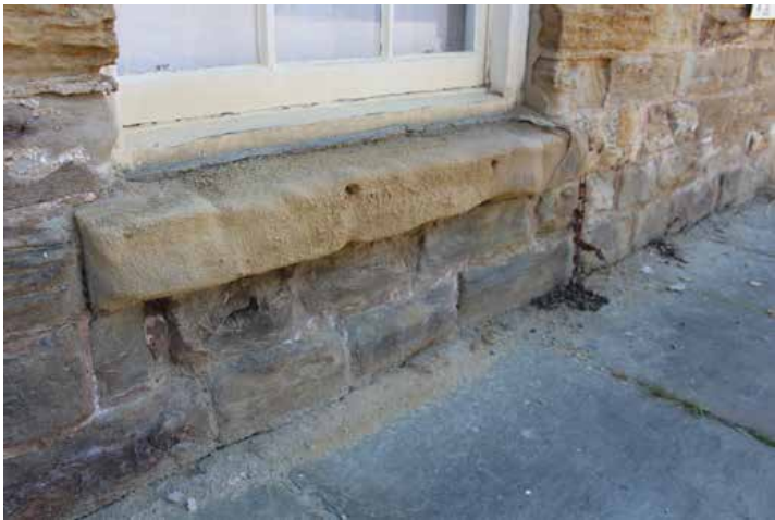
Building 13, deteriorated stone window cill
