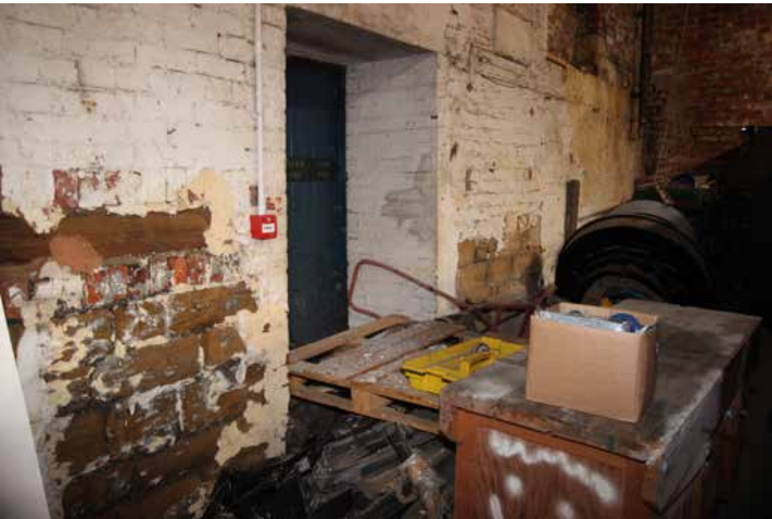
Building 20, high moisture levels in stonework walls
