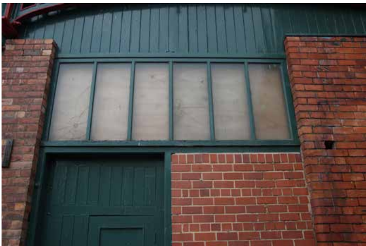
Building 20, cracked panes of glass in fanlight
