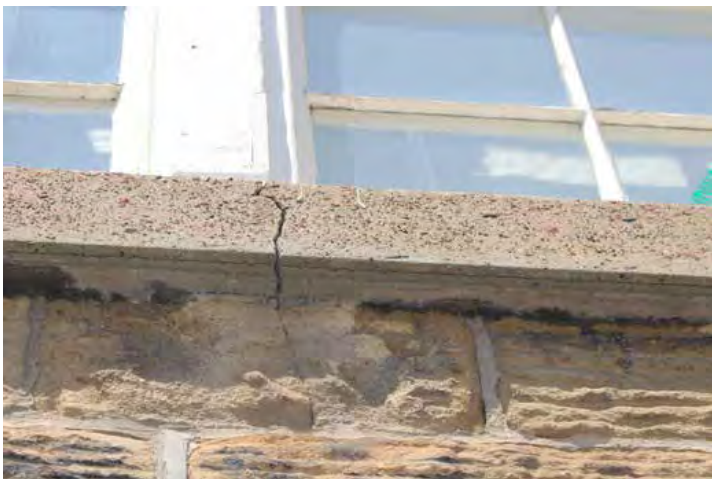
Building 13, cracked concrete window cill
