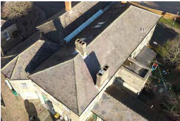
Building 13, drone photo showing slipped slates and other roof defects
