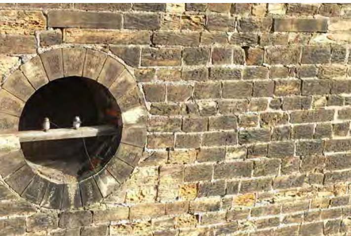
Building 20, heavily open joined stonework at high level
