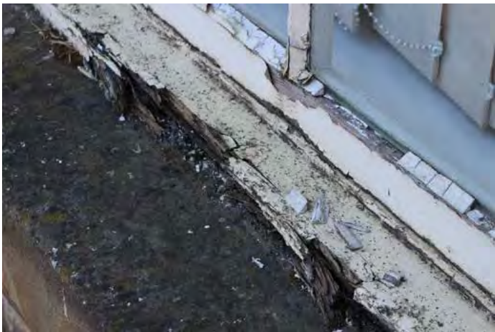
Building 13, window bottom rail in need of replacement
