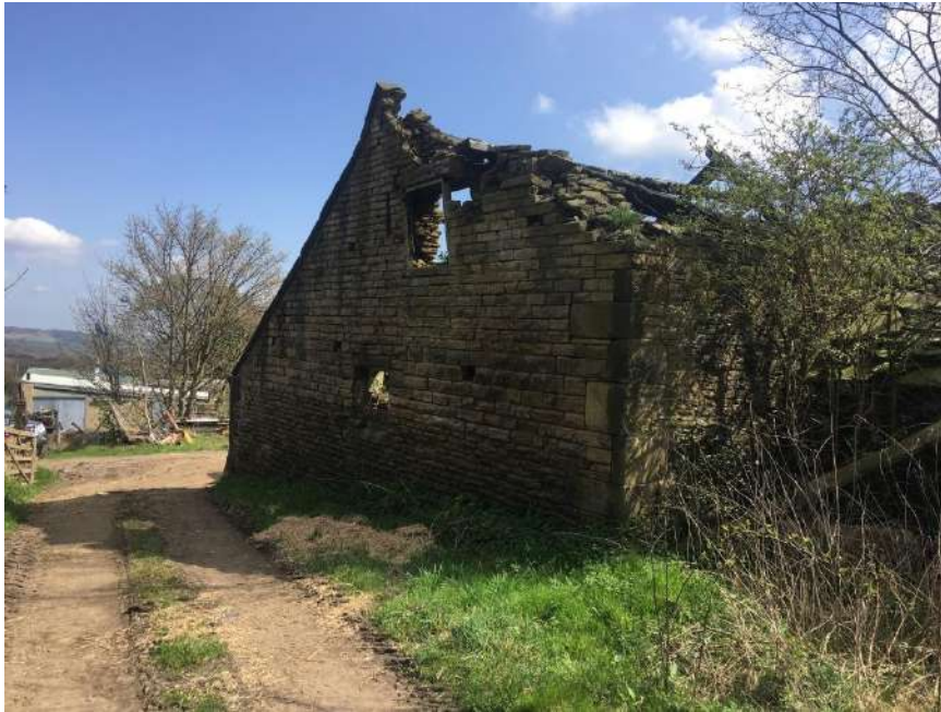
Gable and verge collapse of Unit 1
