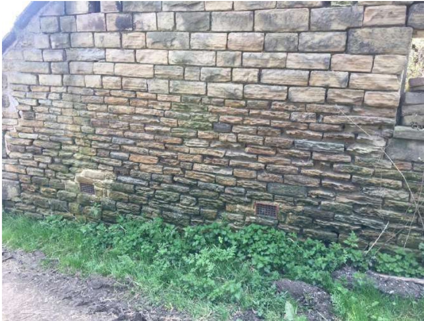
Sandstone walling to Unit 1 eroded at low level
