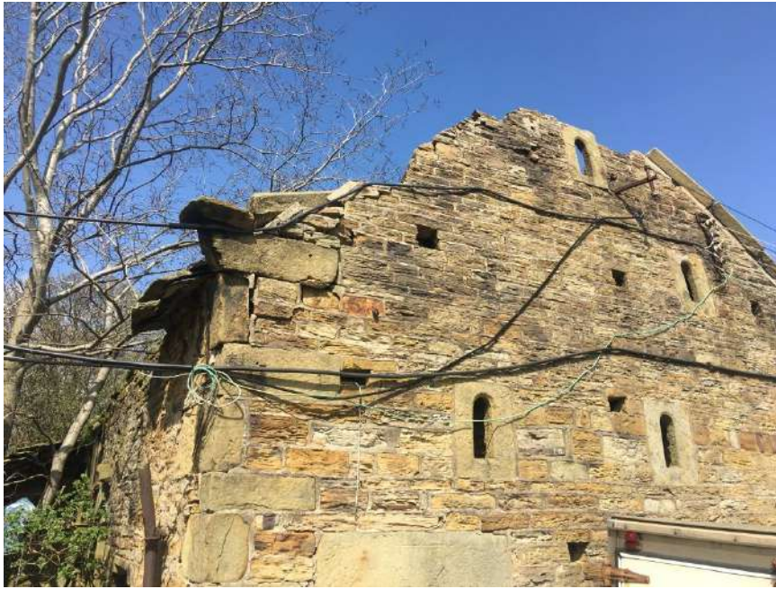
South gable to Unit 1 showing collapsed peak
