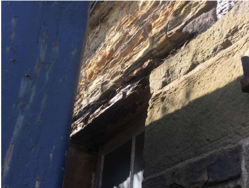
Rotten window head to front of Unit 2
