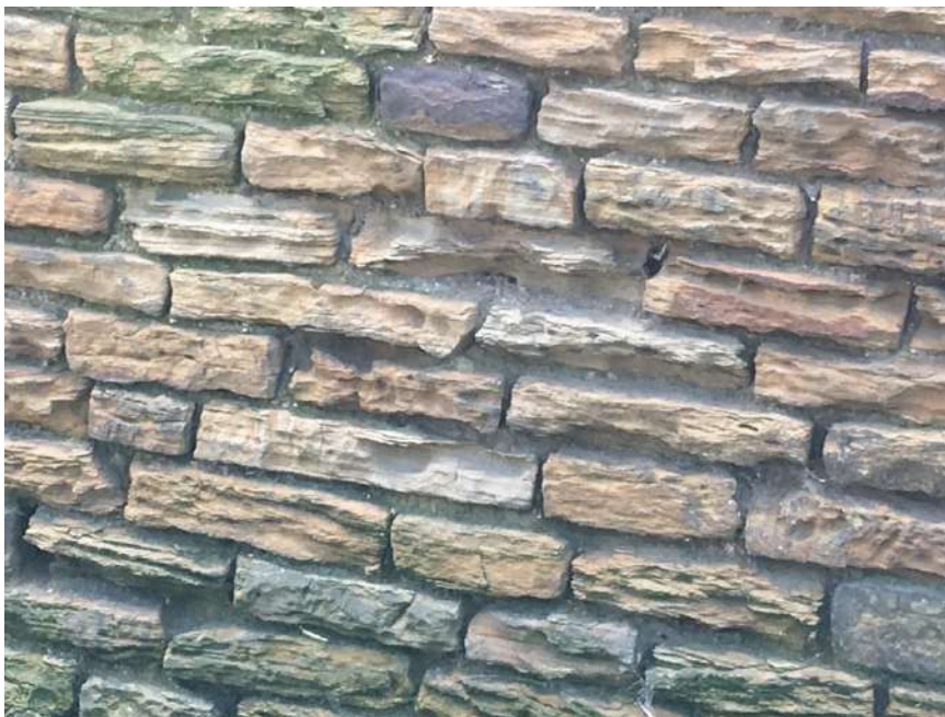
Close up of eroded sandstone to Unit 1
