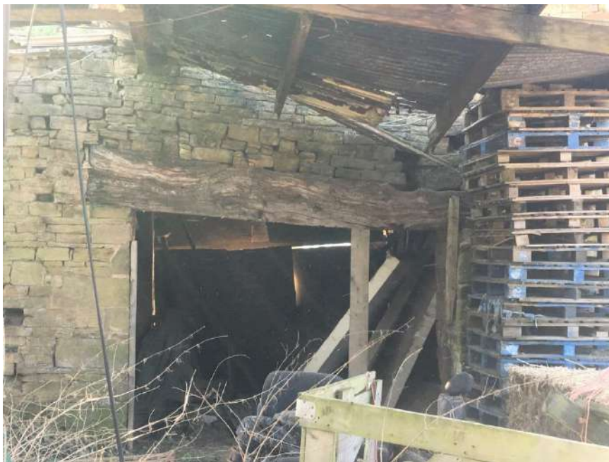
Pallets propping roof to dilapidated perpendicular agricultural pole building (to be removed) to East of Unit 3
