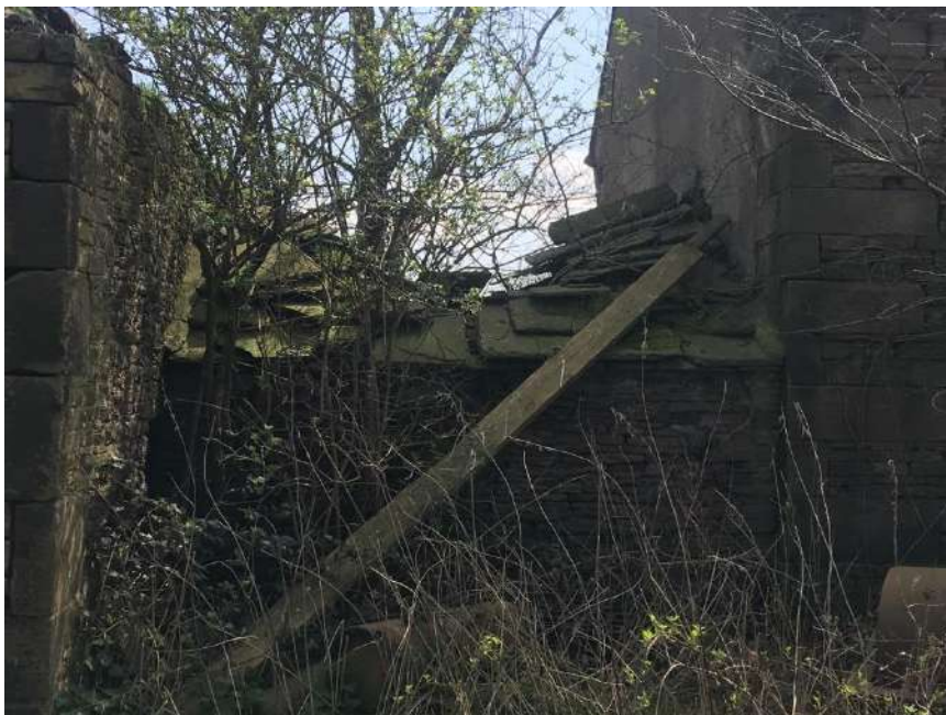
Close up of collapsed duo pitch building between Unit 1 & Unit 2 (viewed from North)
