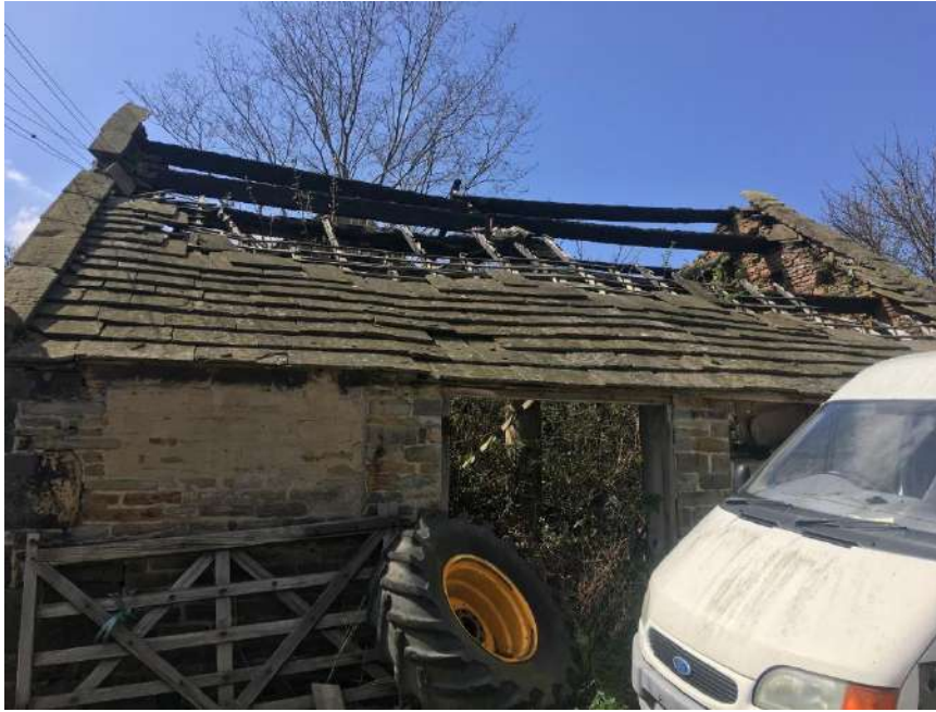
Unit 1 front (East) 50% of front roof slope lost due to fire
