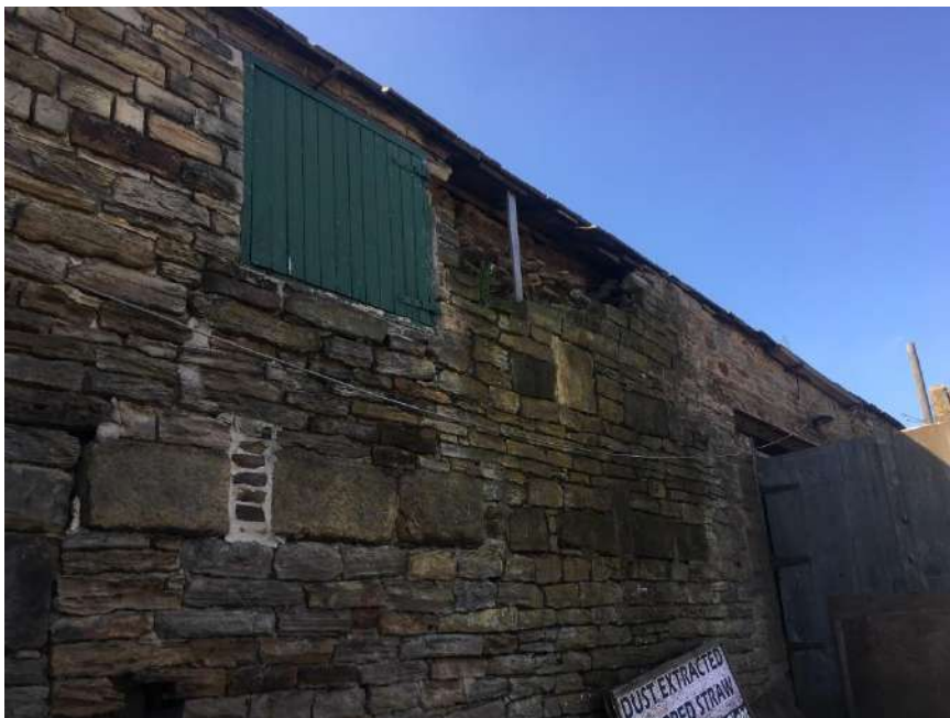
Masonry displacement at eaves level to LHS of principle opening to Unit 3
