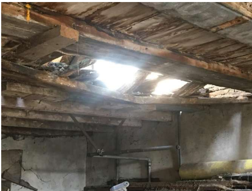
Fractured floor joist to Unit 2
