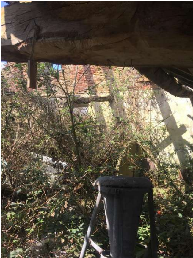
Internal shot of Unit 1 note red coloured masonry showing effects of fire
