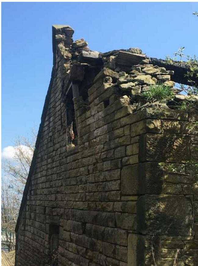
Leaning peak of partly collapse gable peak to Unit 1
