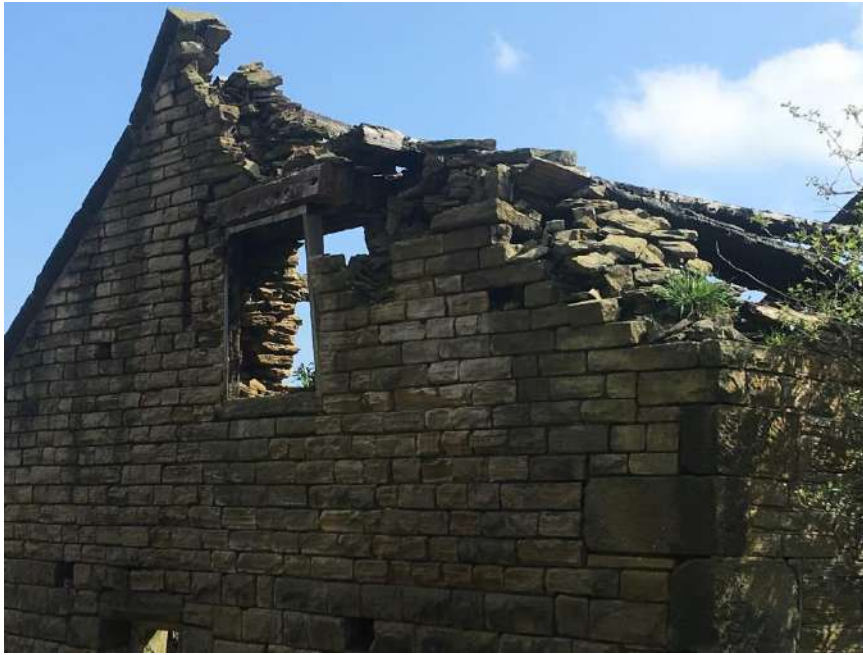
Closer view of gable and verge collapse to Unit 1
