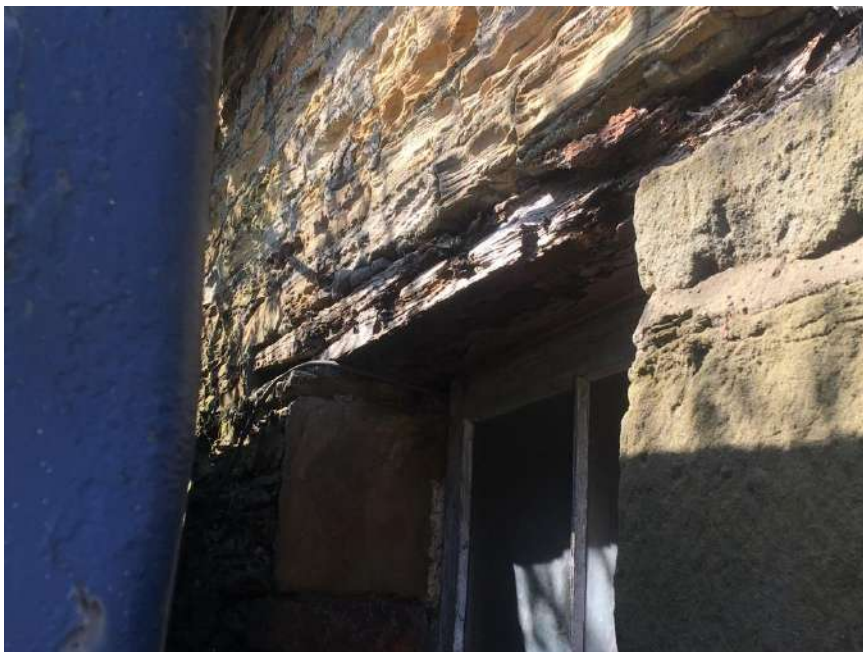
Rotten window head to front of Unit 2
