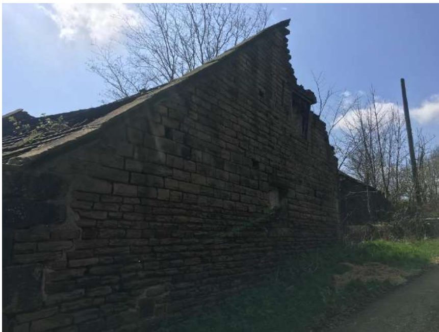
Partly collapsed North gable peak of Unit 1
