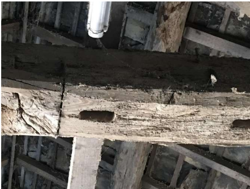
Insect infestation to bottom chord of truss within Unit 3
