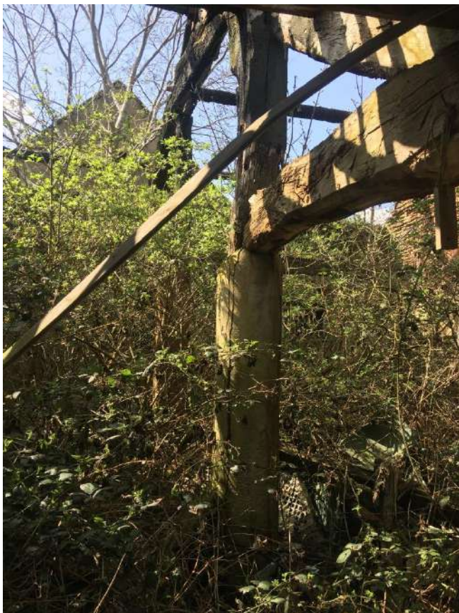
Internal photo of Unit 1. Masonry prop to remains of fire damaged truss
