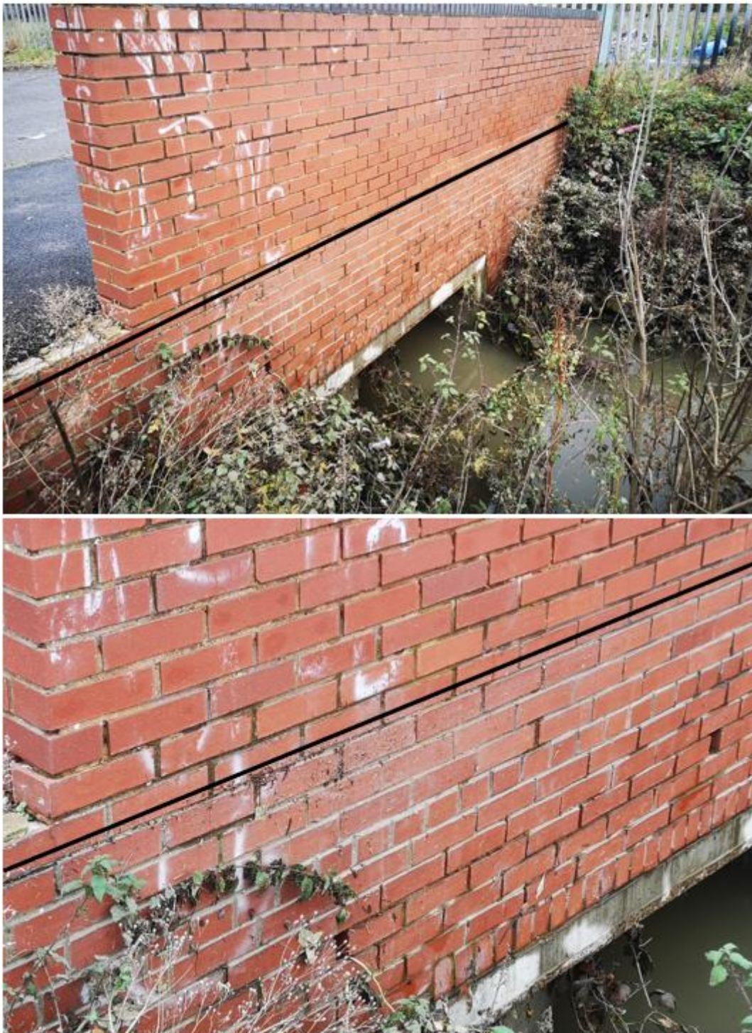
Figure 9: Bulling Dyke wrack mark downstream face of Valley Road access bridge
