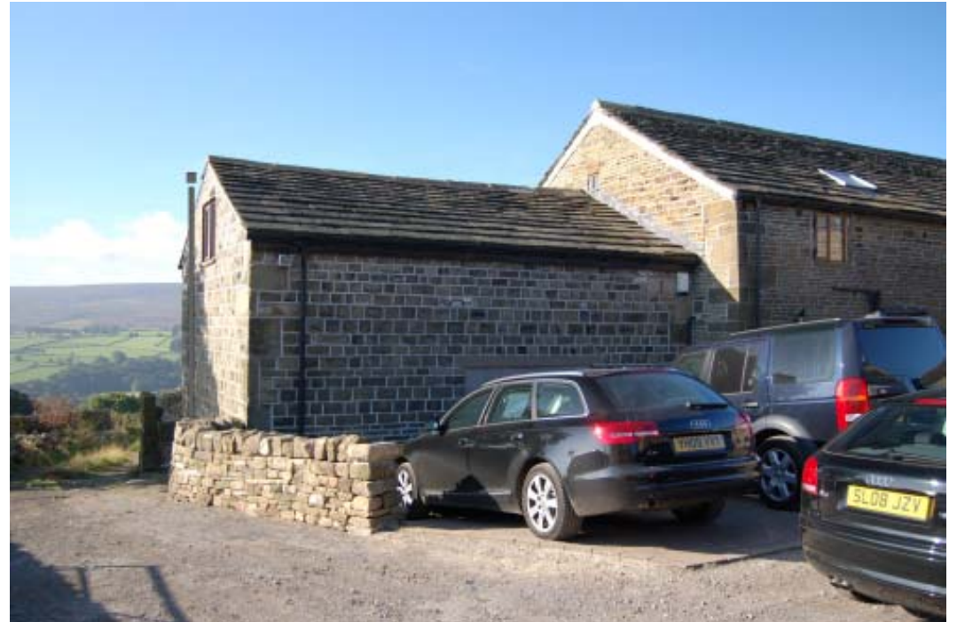
Showing the flue
