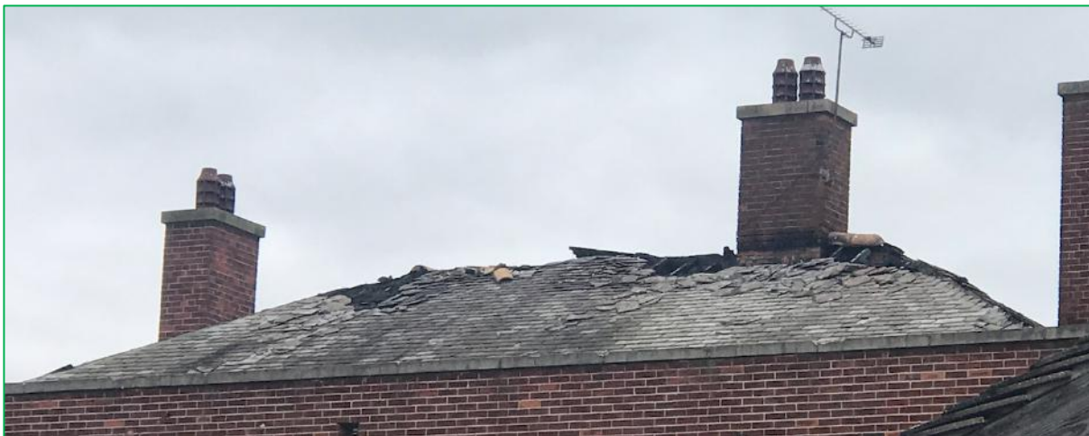
Showing lifted and missing slates on the west elevation of the building
