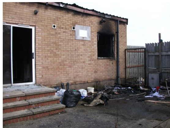
Image 3: The Fleets, currently subject to severe vandalism – Barnsley College propose to secure the site and monitor, allowing neighbours to feel safe.
