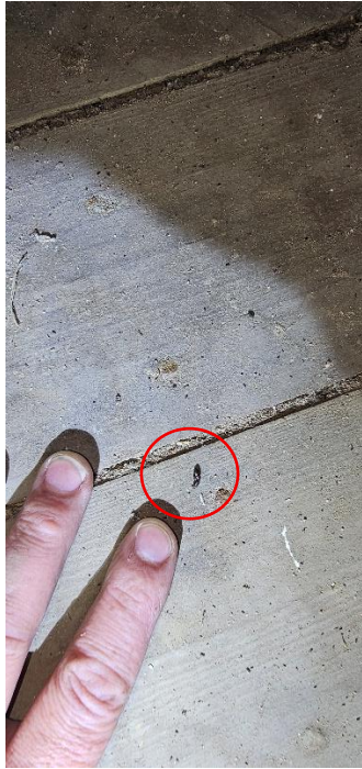
Photo 1 close up of bat dropping 6/08/2026
