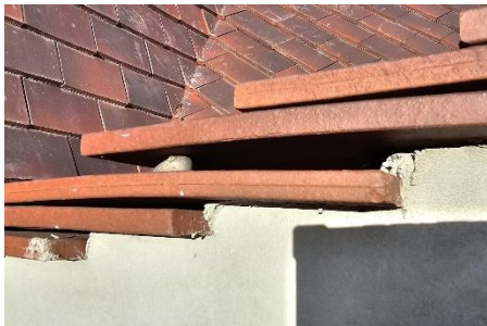
Figure 8-12: Gaps under tiles along verges
