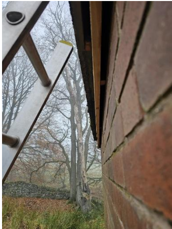
Figure 8-9 Gap behind fascia boards
