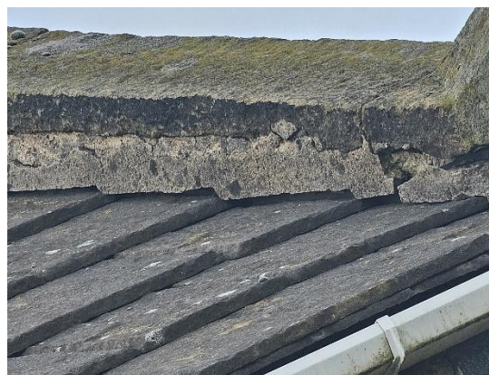
Photo 10 Roost C gap in mortar under parapet
