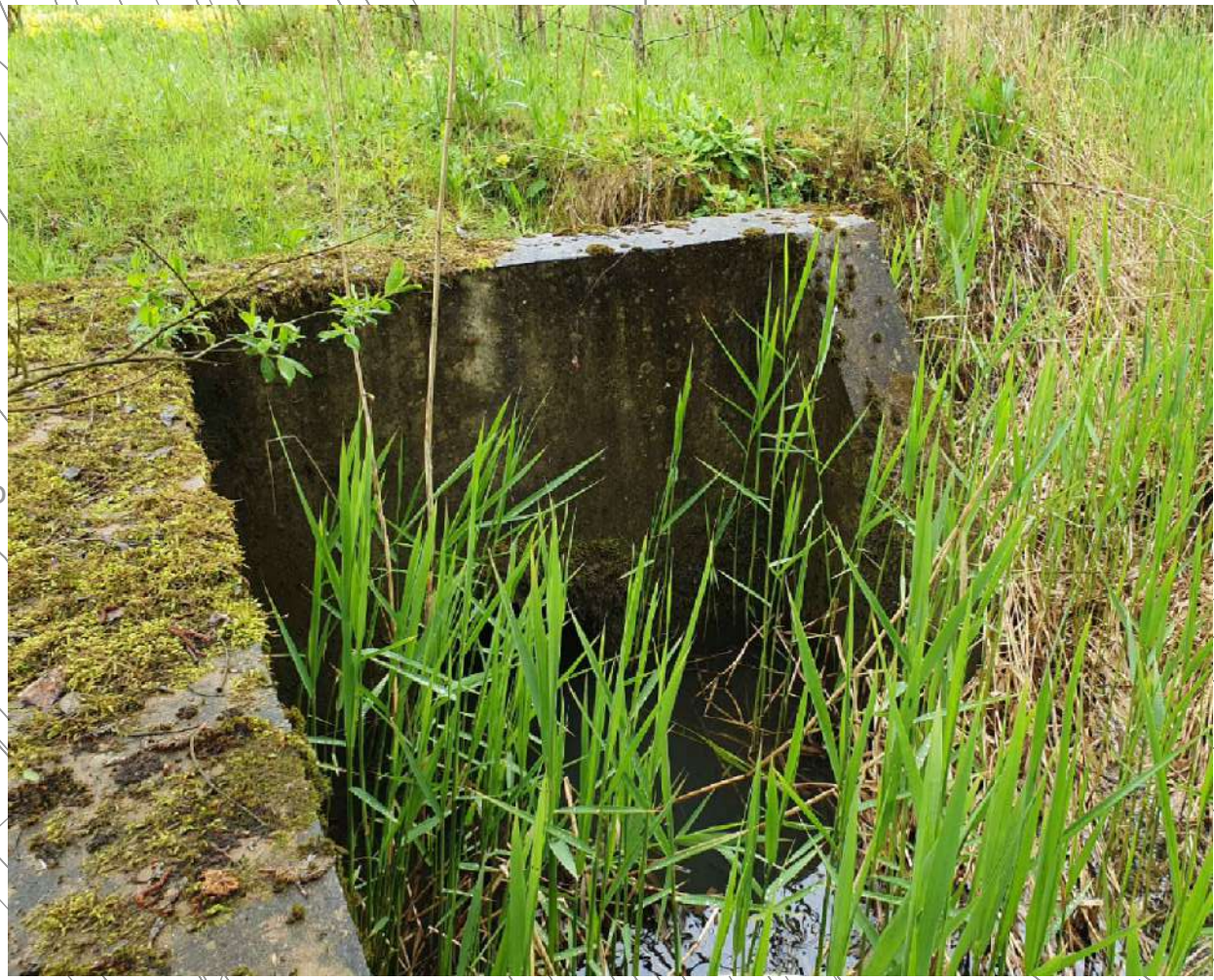
CONCRETE HEADWALL WITH CIRCA 0.6m PIPE FROM ASOS DEVELOPMENT SIGNIFICANT FLOW (17.05.21)
