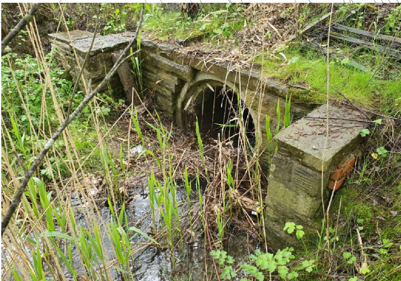
STONE HEADWALL WITH CIRCA 1.05m PIPE SIGNIFICANT FLOW (17.05.21)
