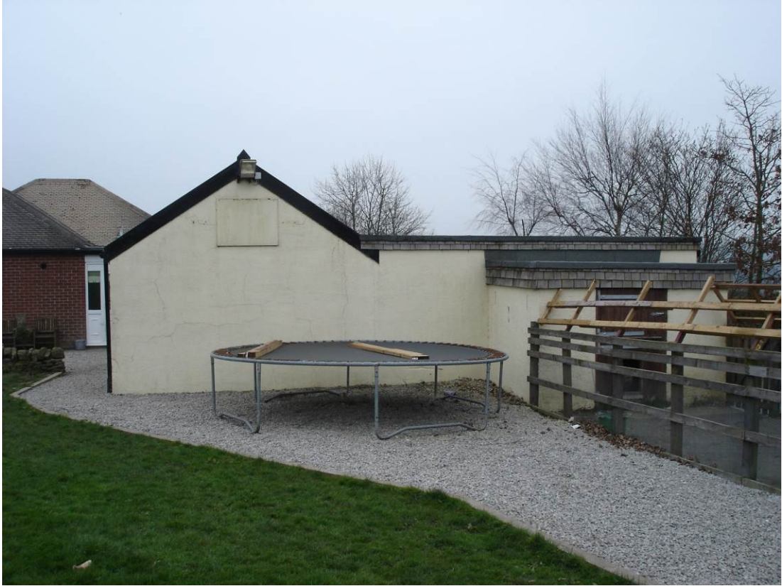
07. Further view of north east elevation of outbuilding and store at rear.
