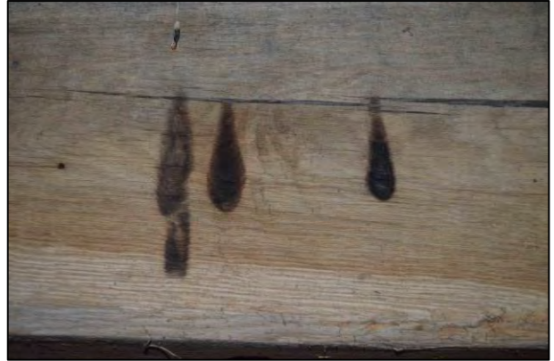
Figure 31: Detail of taper burn marks on loft joist
